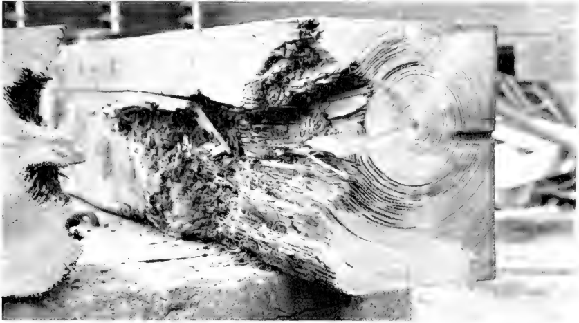
Fig. 9. —Termite injury to the frame of a large school building. In this case the entire sill had been honeycombed and largely destroyed by termites, which had built their tunnels in it.
