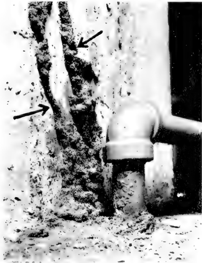
Fig. 4.—Very large termite tubes extending through a poorly constructed concrete floor over a concrete basement wall.
