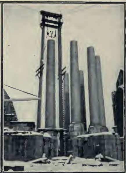
The eight giant pillars of the choir and the derrick used in hoisting them into place.
