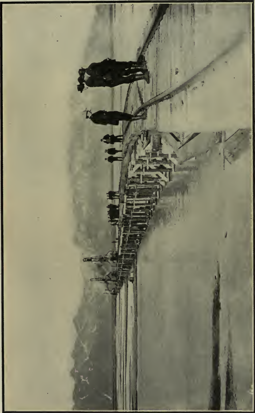
Stretch of temporary trestle over the silt flats of the Copper River delta.
