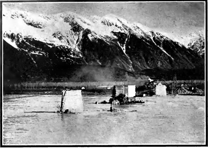
Concrete piers for the Miles Glacier bridge across the Copper River, made strong enough to withstand great ice pressure.
