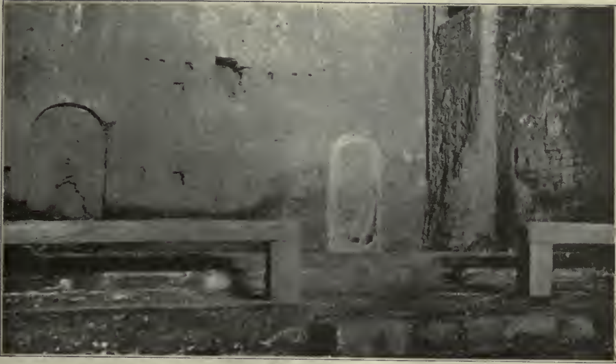
Interior of Church: The Altar.—The large hole, high in the center of the wall, was made by treasure seekers who thought to discover gold and jewels secreted beneath the beam-end on which rested the great silver Crucifix long since removed.
