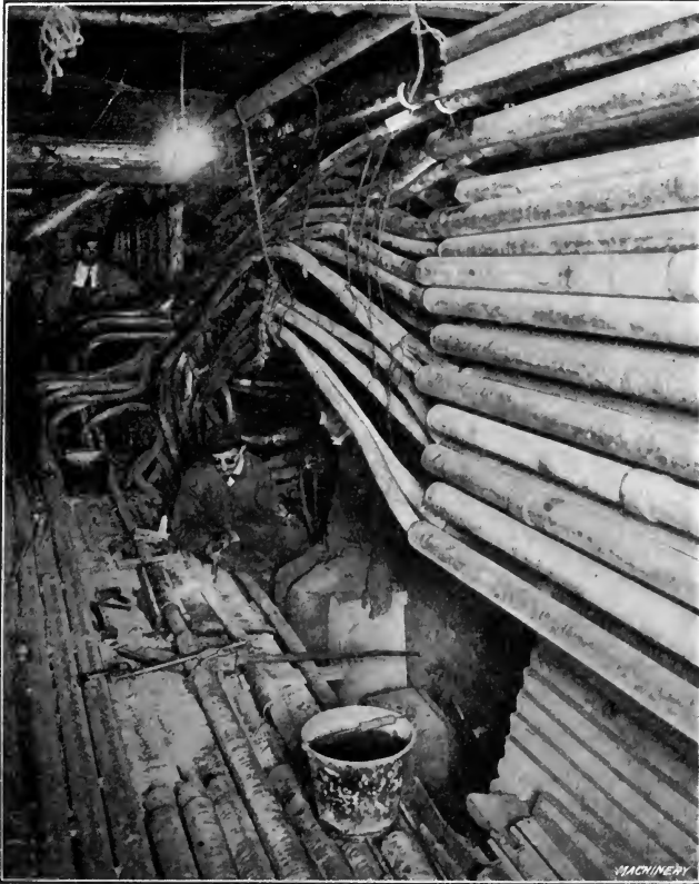
Fig. 1. Oxy-acetylene Torch being used for Cutting away Iron Armor of Lead-covered Telephone Cables
