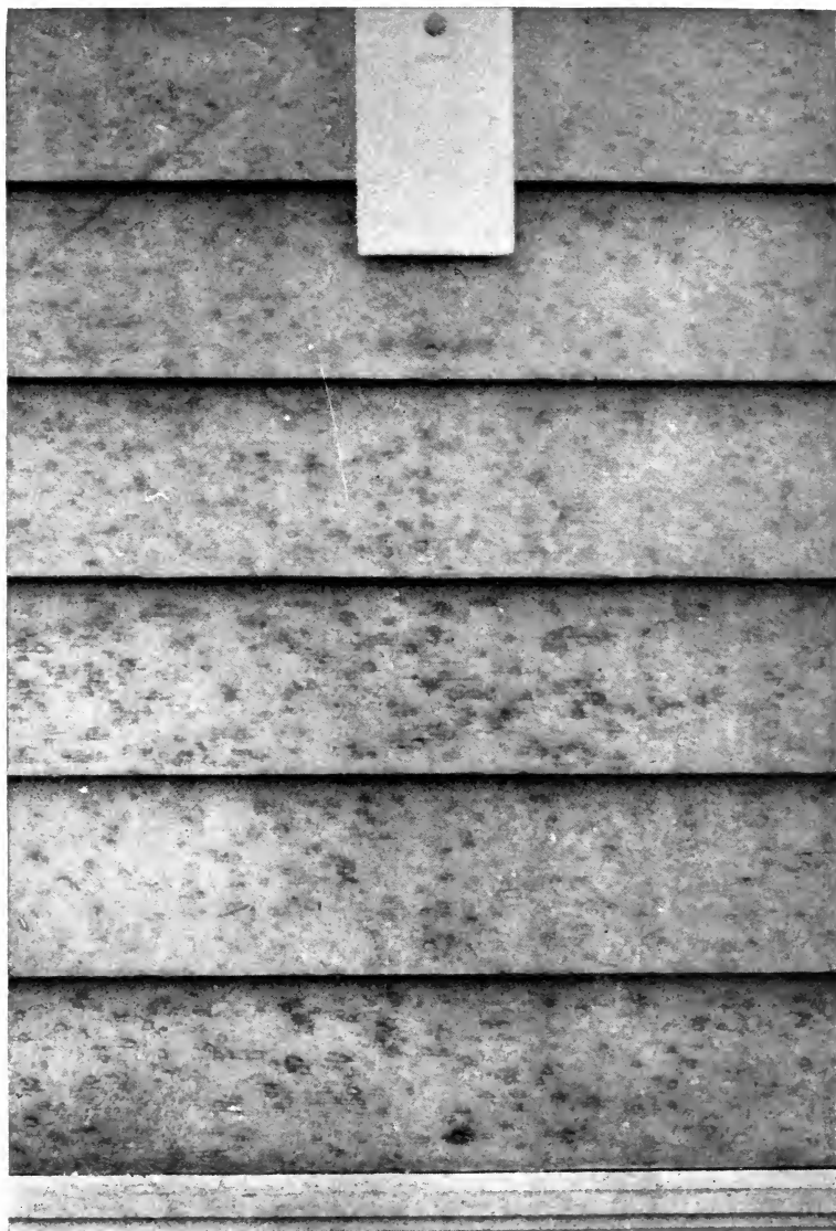
Hail-stone Abrasions on House Repainting Tests
