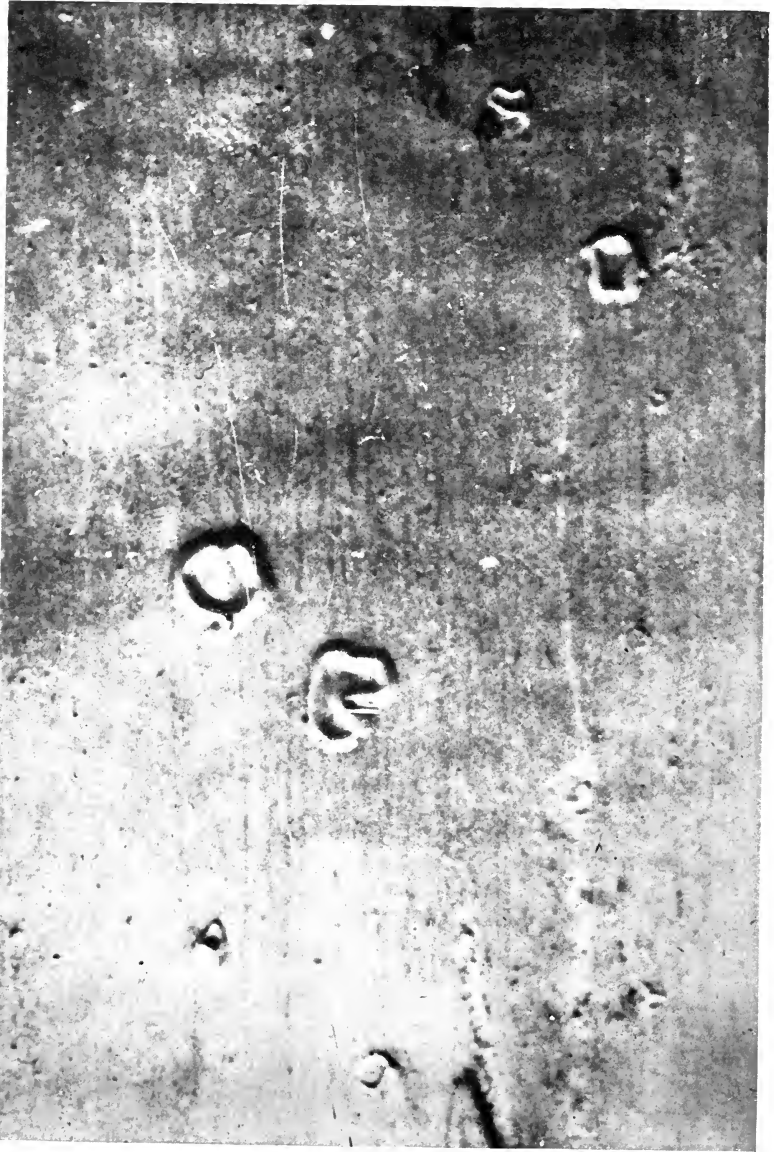
BLISTERING. — Type of Decay Exhibited by Improperly Made Paint (magnified view)
