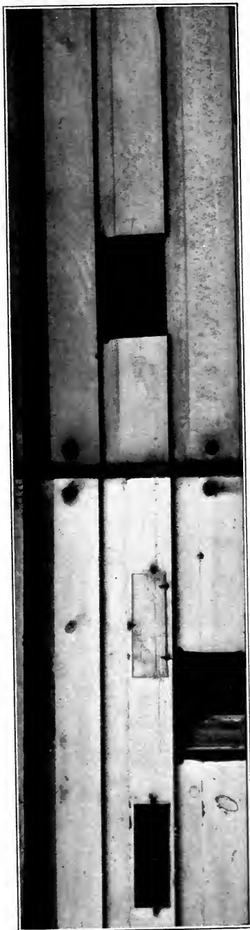
Darkness of Corroded White Lead
