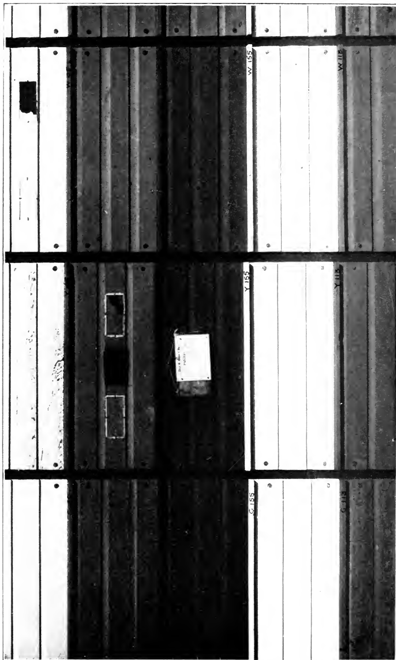
Panels on Atlantic City Fence Two Lower Sets of Panels are Painted with Combination Pigment Paints. Excellent Results shown
