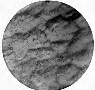
23. Section 65 on 1908 Fence. Showing Early Break-down of Corroded White Lead
