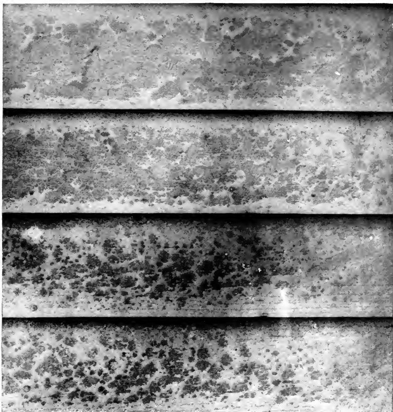
Peculiar Crystallization Effect on Section 41. New Special Fence Paint Applied During Cold Weather
