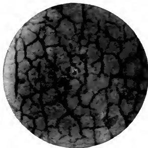
13. Panel No. 34, Formula 23, on 1907 Fence. Deep Checking on Corroded White Lead
