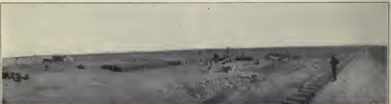
This Is One of the Cement Pipe Plants, Making the Concrete Conduits on the Ground, for Carrying the Irrigating Water to All Parts of the Palmborg Colony
