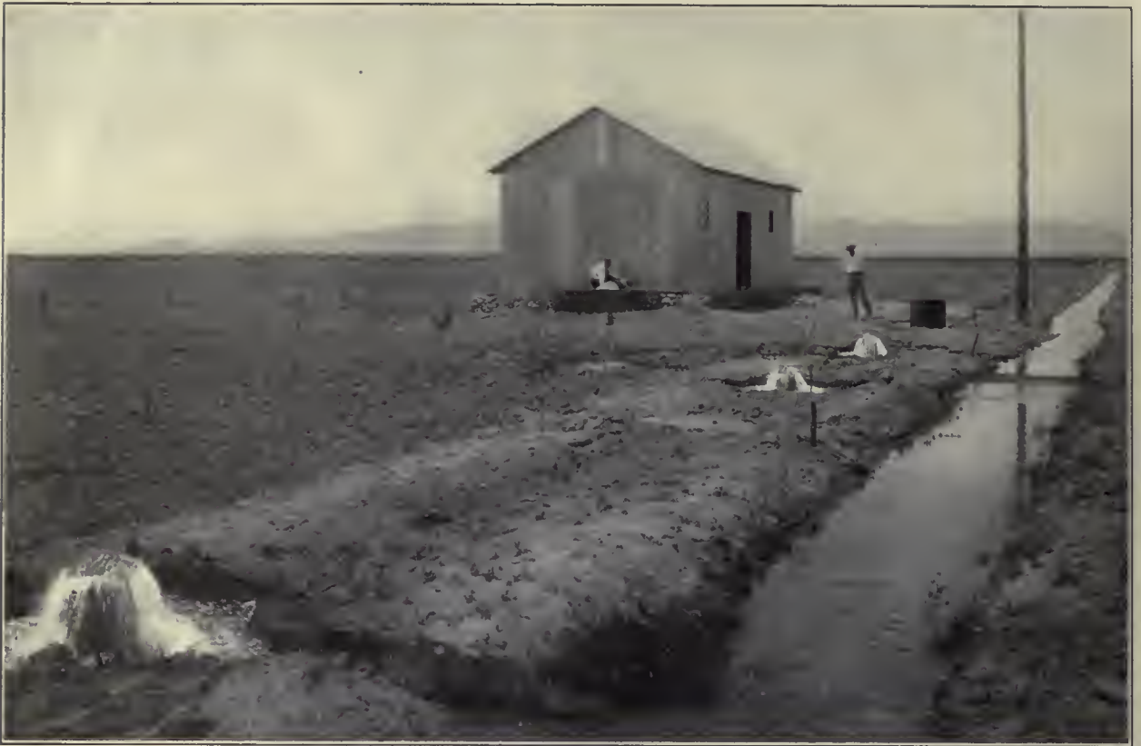
One of the Pumping Plants Showing Canal and Hydrants
