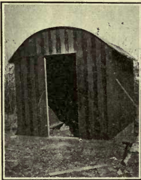
A well constructed fumigating house. It is built of tongue and grooved lumber and cleats cover the joints on the outside
