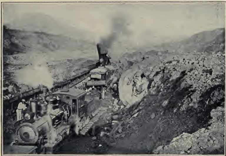
STEAM SHOVEL AT WORK ON THE SITE FOR THE PEDRO MIGUEL LOCKS.
