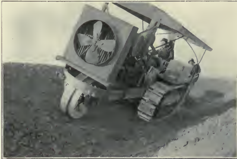
Caterpillar tractor with two-furrow ditching plow building irrigation ditch and levee at the same time.
