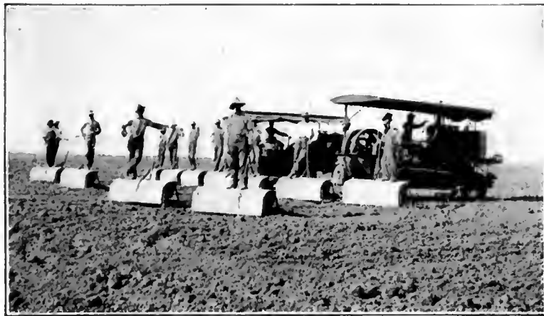
A tractor pulling a battery of scrapers. Grading and leveling land ready for water.
