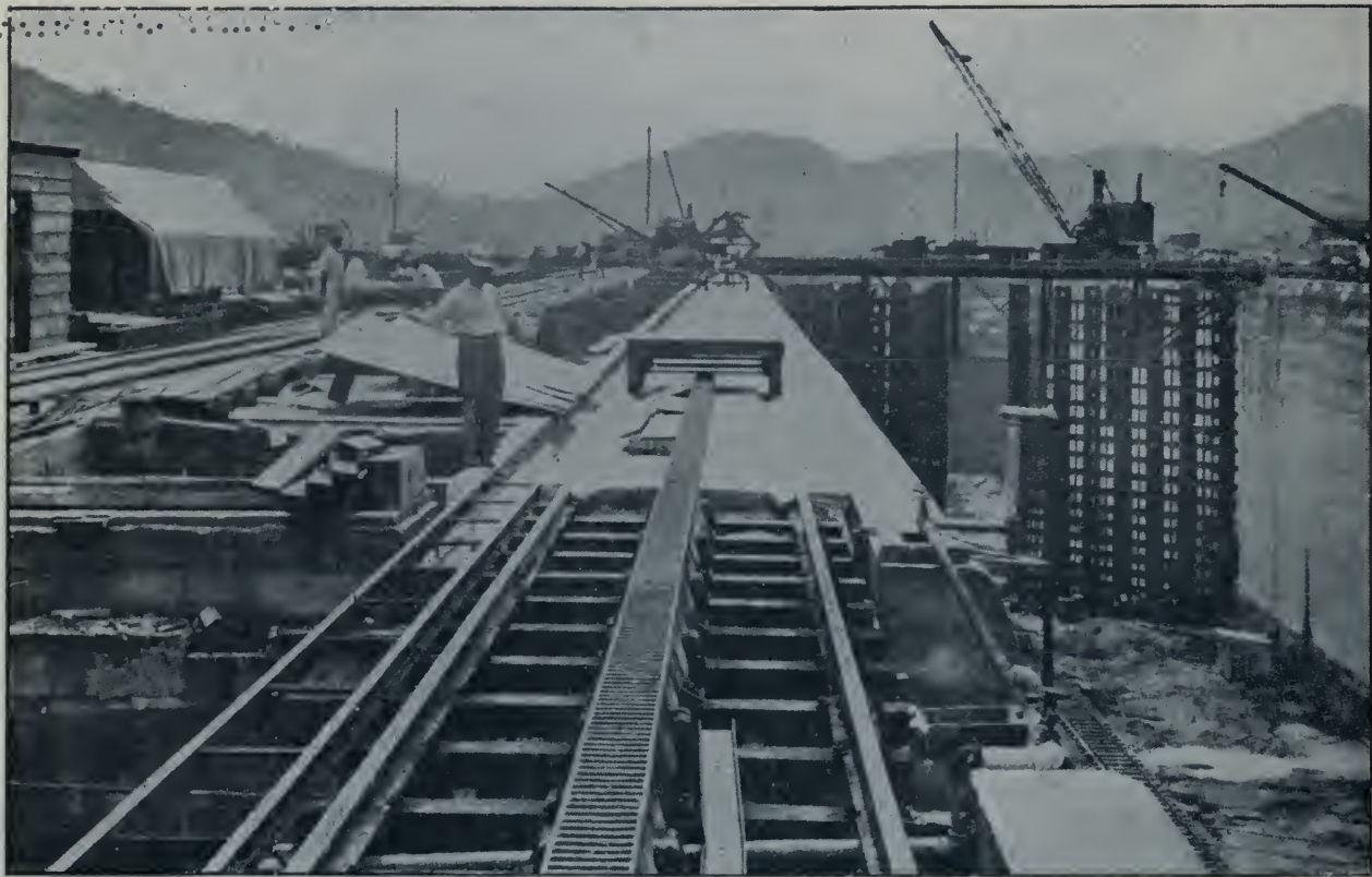
Pedro Miguel Locks, Detail of Construction of Electric Towing Locomotive Rack Track. All Vessels Will Be Towed by Electricity Through the Canal.
