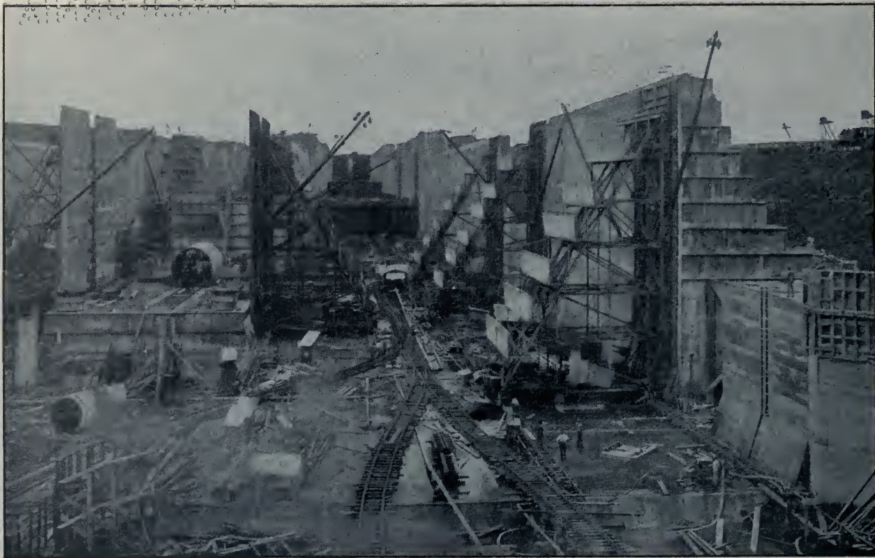
Gatun Lower Locks Looking South from Cofferdam, Showing West Chambers of Upper and Middle Locks, as They Appeared on November 9, 1911.
