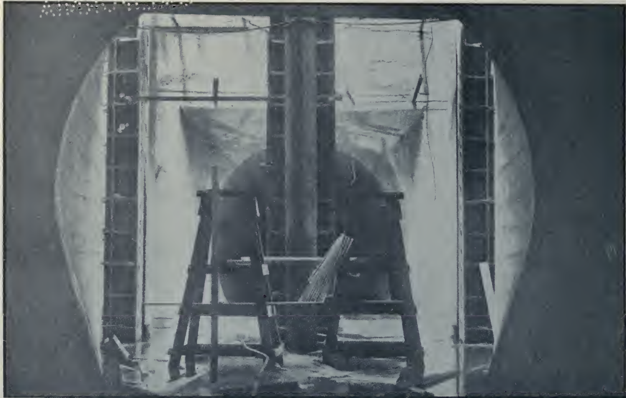
Miraflores Upper Locks, Center Wall Culvert, Showing Stoney Gate Castings in Place. Photographed June 23, 1912.
