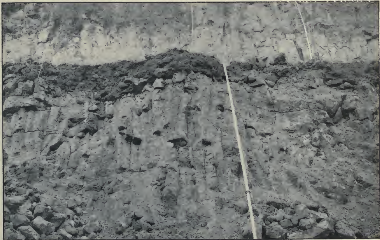
Columnar Structure in Hardened Flows of Mud Lava. This Jointing Afforded Passages for Seepage Water Which Tended Largely to Promote a Large Slide Just North of La Pita.
