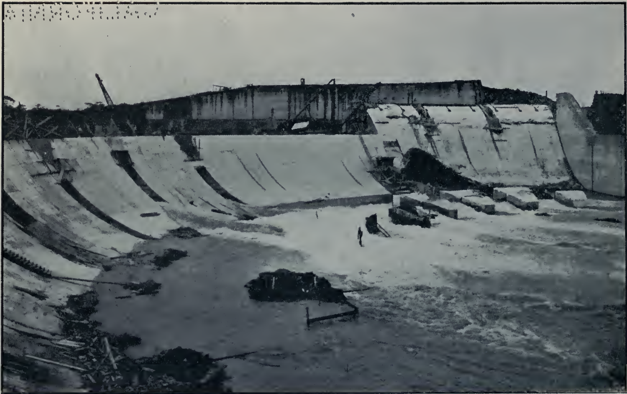
Gatun Spillway Looking Southwest, Showing Downstream Face of Ogee Dam, as it Appeared June 6, 1912.
