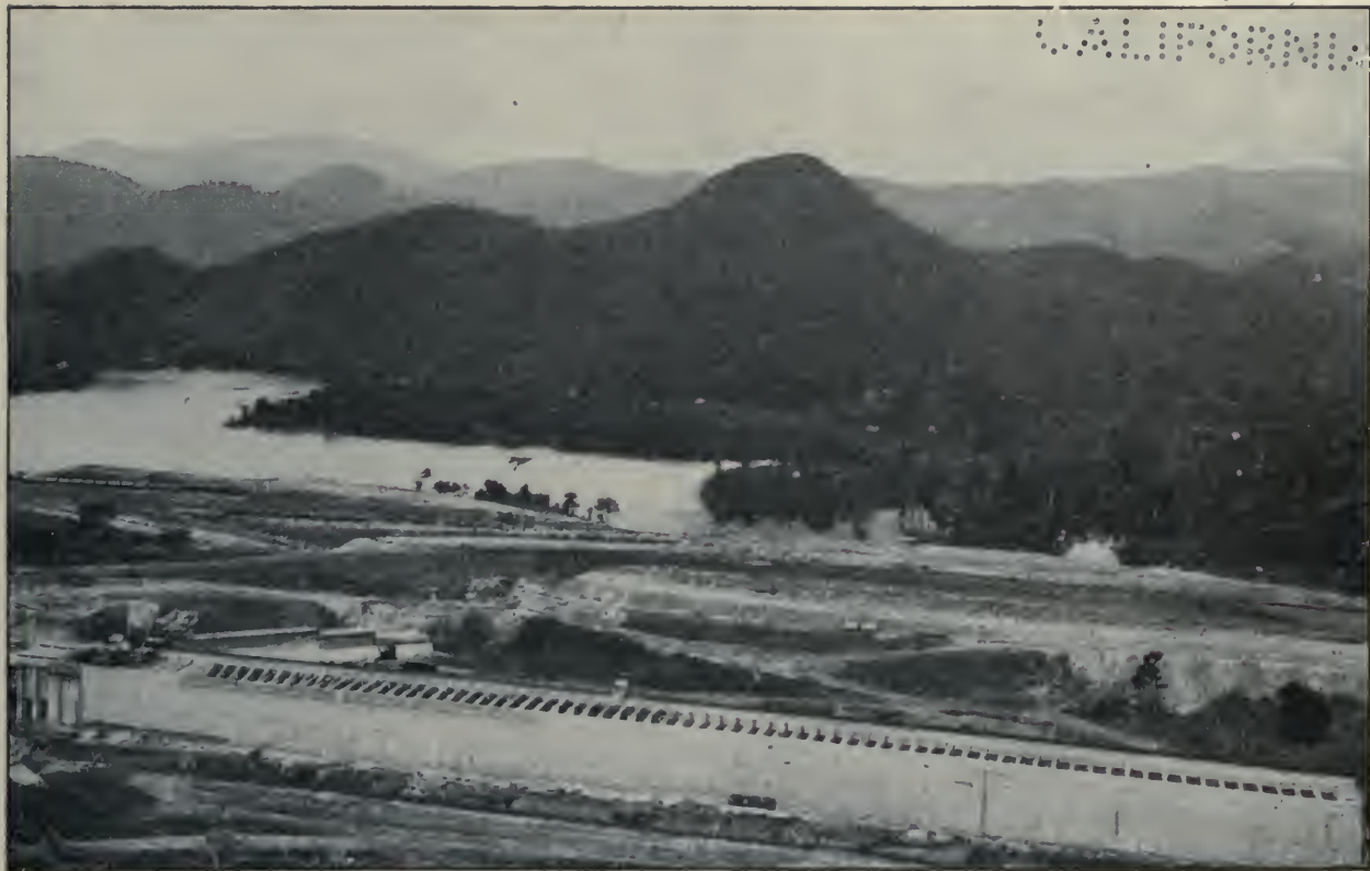
Pedro Miguel Locks. Bird's-eye View of North Approach Wall from Hill at East End, as It Appeared July 28, 1912.
