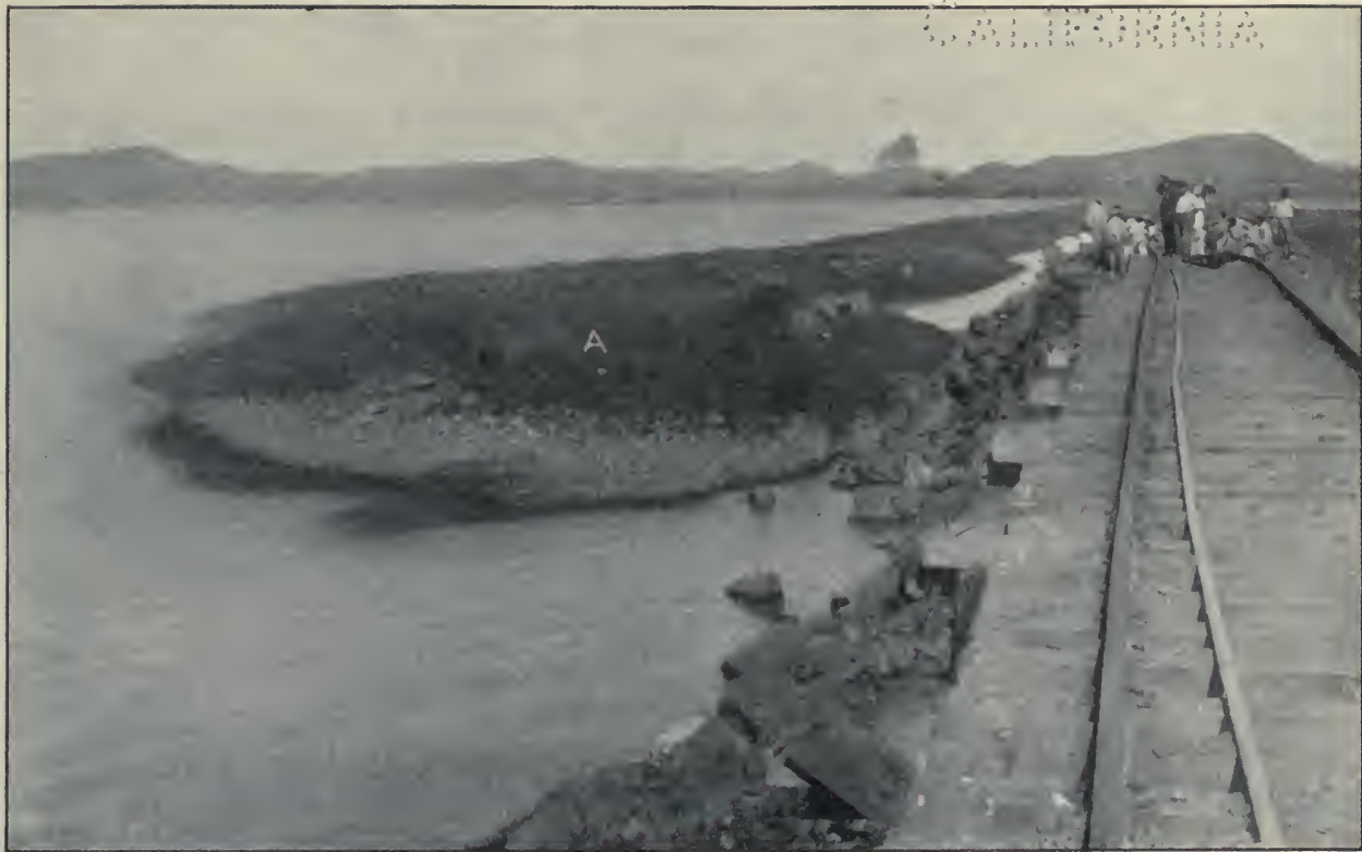
South End of Naos Island Dump, 4,000 Feet from Island. Center at "A" Is 80 Feet from Track and 25 Feet Above the Original Bottom. Elevation of Trestle, +14. Photographed in December, 1911.
