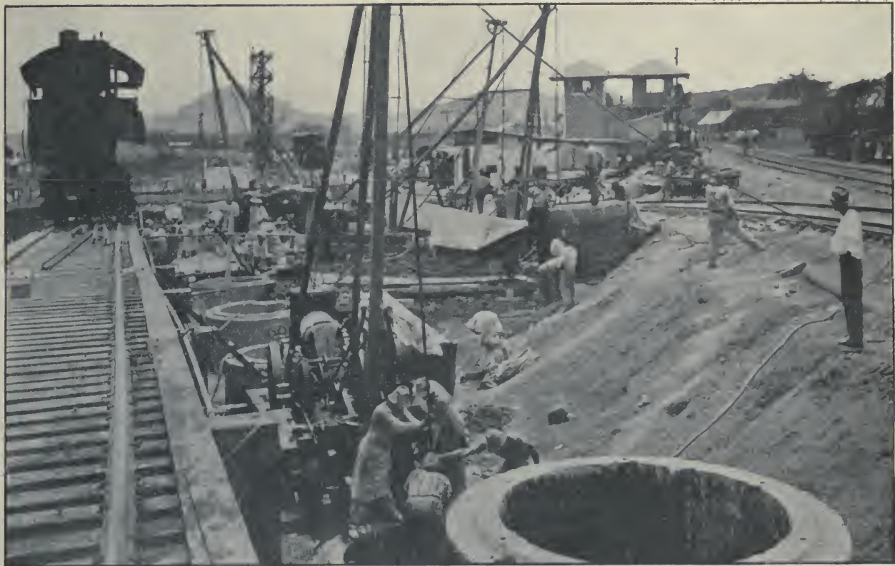
Miraflores Locks. Sinking Caissons for Foundation of North Approach Wall, Looking North, June 14, 1912.
