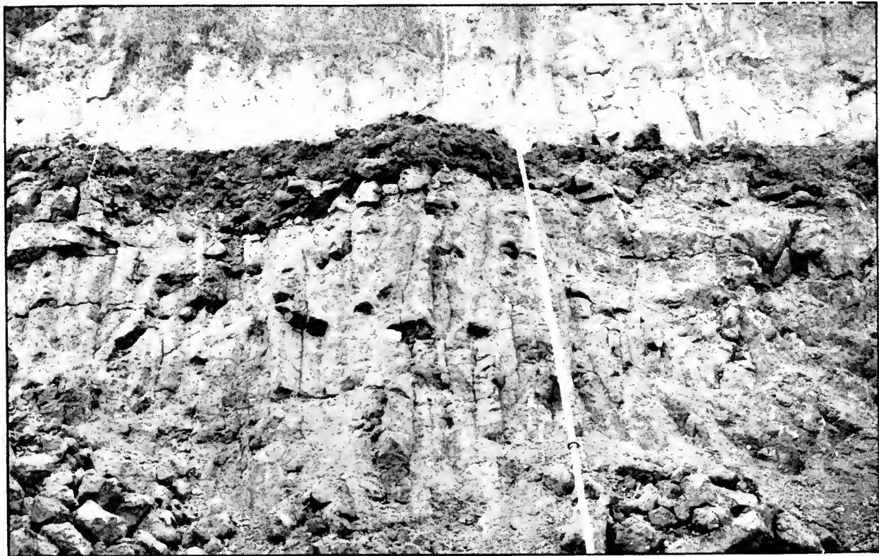
Columnar Structure in Hardened Flows of Mud Lava. This Jointing Afforded Passages for Seepage Water Which Tended Largely to Promote a Large Slide Just North of La Pita.
