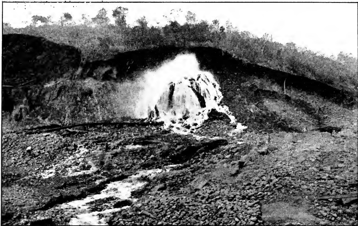
Stripping Cocoli Hill Adjacent to Canal Prism. Photographed March 21, 1912, and Showing the Method of Hydraulic Excavation.
