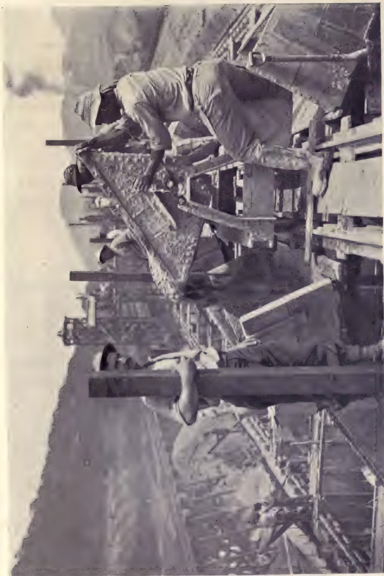
CONSTRUCTING THE APPROACHING WALL OF CONCRETE AT THE PEDRO MIGUEL LOCKS, JUNE, 1912.
