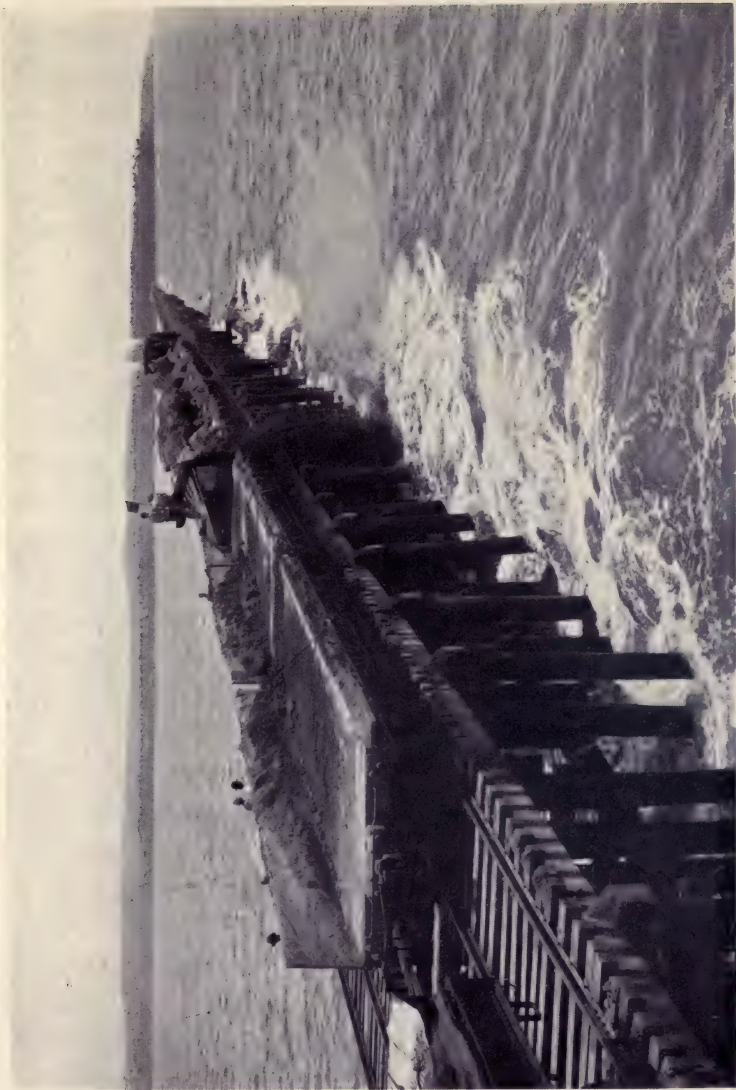
BUILDING THE BREAKWATER TO PROTECT THE ATLANTIC ENTRANCE TO THE CANAL. JULY 21, 1911.
