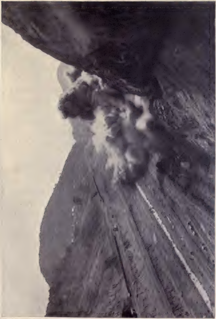
CULEBRA CUT AT CULEBRA: VIEW LOOKING SOUTH; BLASTING ROCK ON CONTRACTORS' HILL, JANUARY, 1912.
