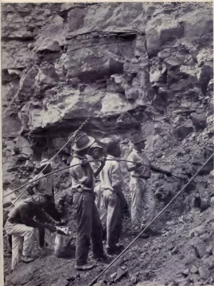
HAND DRILL GANG BORING HOLES FOR DYNAMITE TO BLAST MOVING FACE OF A "SLIDE" IN THE CULEBRA CUT, FEBRUARY, 1912.
