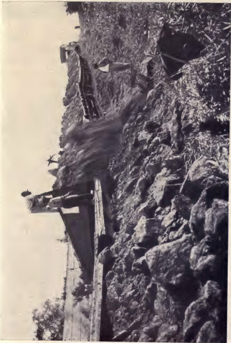
DUMPING "DIRT" FROM CANAL EXCAVATIONS; THE STEEL WEDGE HAULED BY A CHAIN RAPIDLY PUSHES ALL THE DEBRIS ON ONE SIDE.
