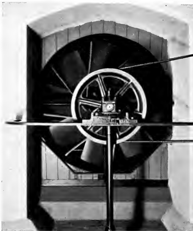
BIG FAN EXHAUSTER, VENTILATING DEPARTMENT.
