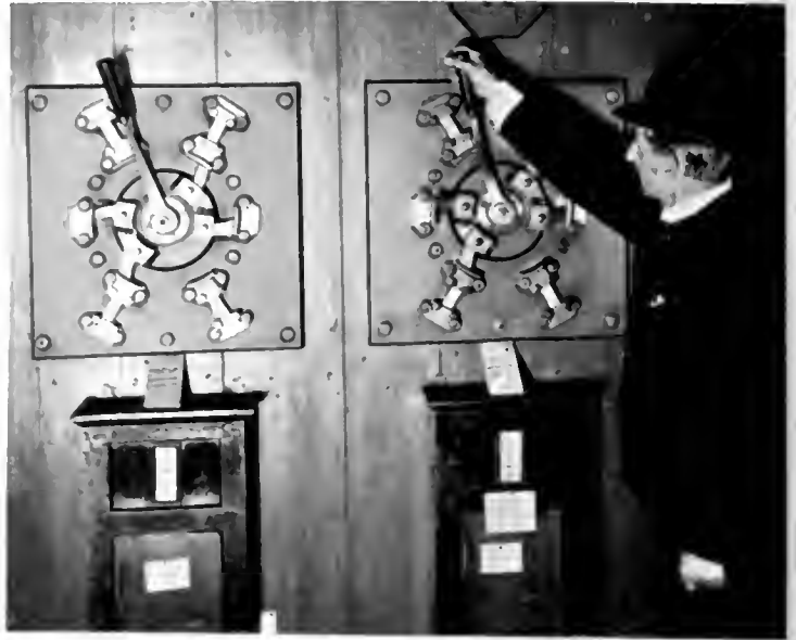
ELECTRIC SWITCHES UNDER THE HOUSE OF LORDS.
