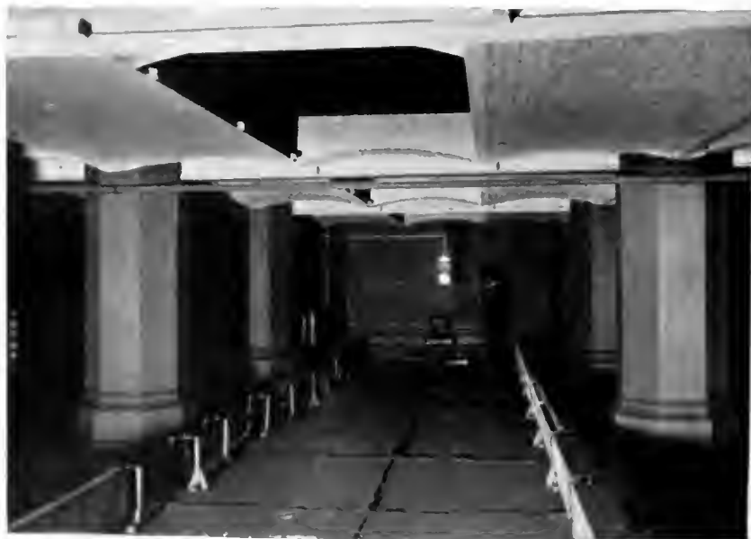
THE RADIATORS UNDER THE HOUSE OF LORDS.
