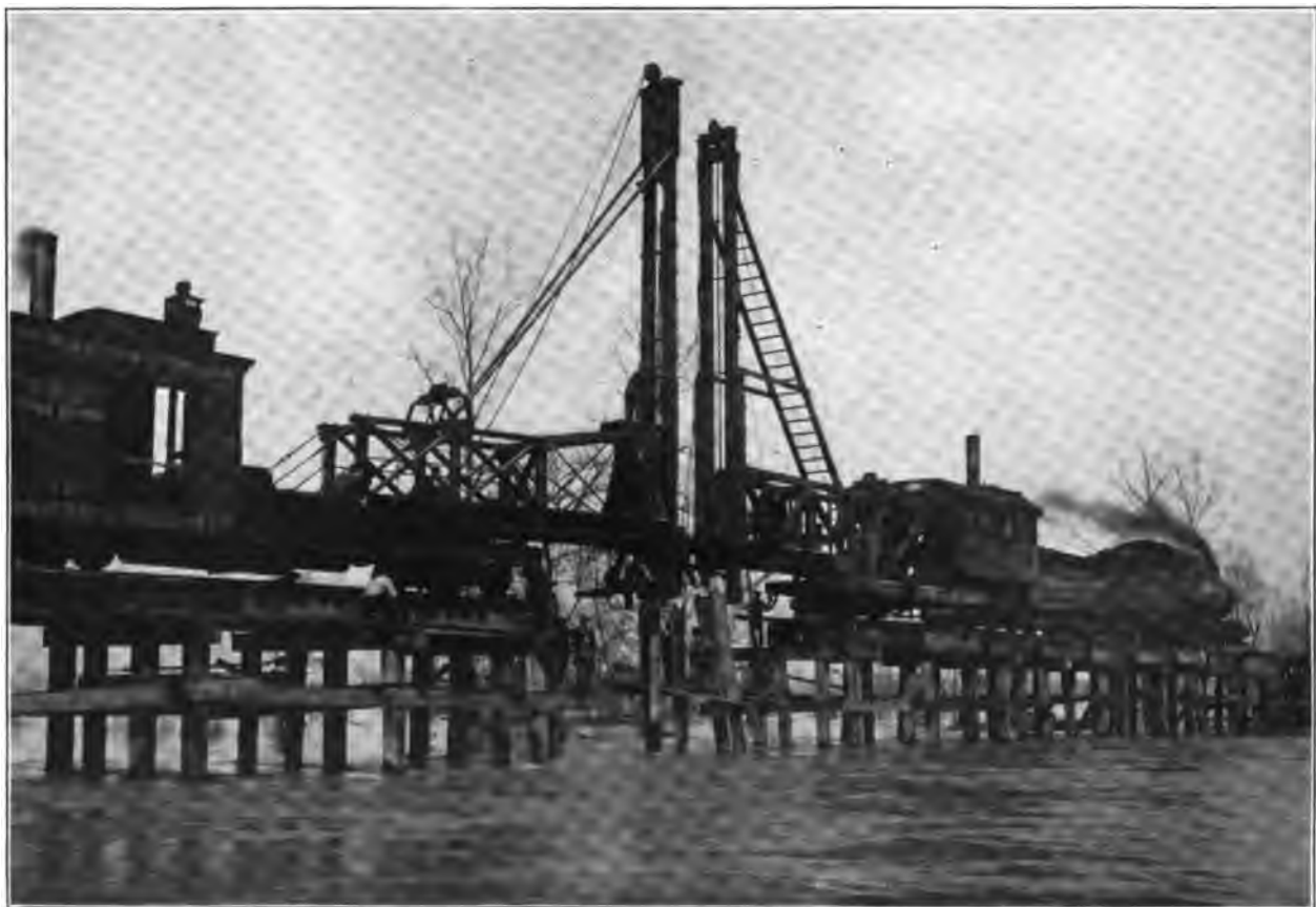
Macksville, Ind. April 2, 1913. Closing the east gap in the St. Louis Division main line.
