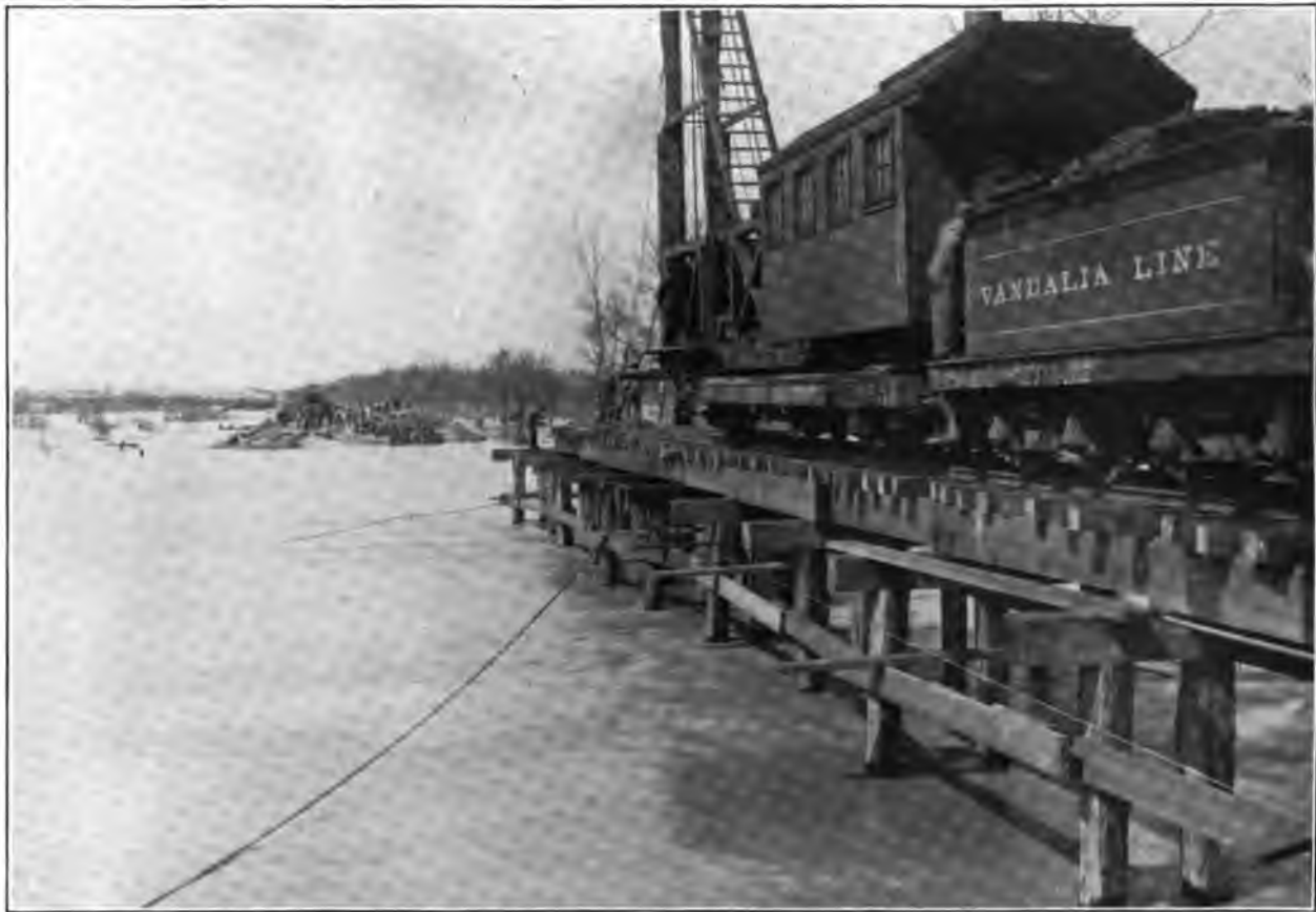
Macksville, Ind. April 1, 1913. Looking west across east gap in St. Louis Division main line.
