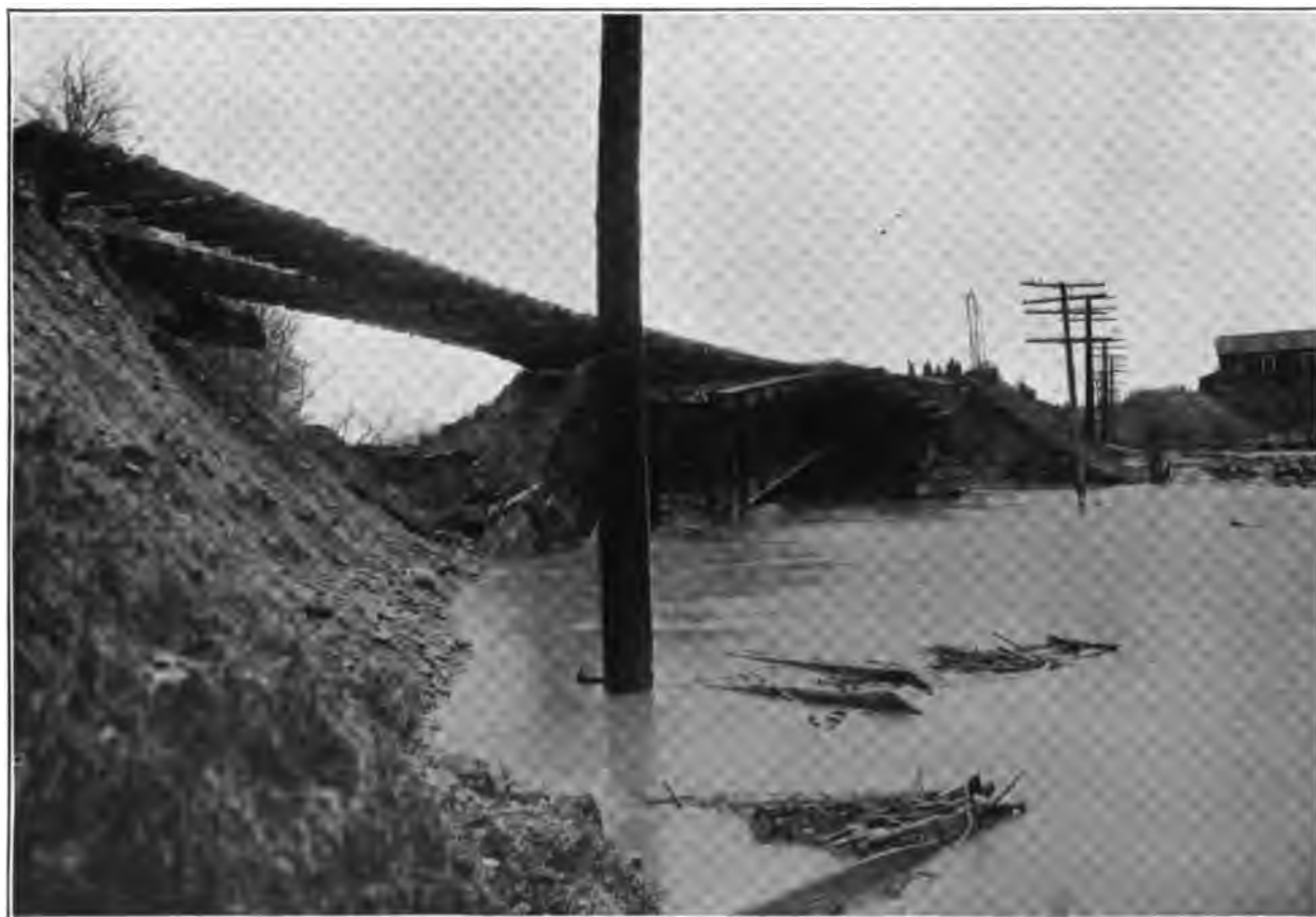
Lucas, Ohio, east of. March 26, 1913. Bridge No. 146, over Rocky Fork, both abutments and about 125 feet of embankment approach destroyed.
