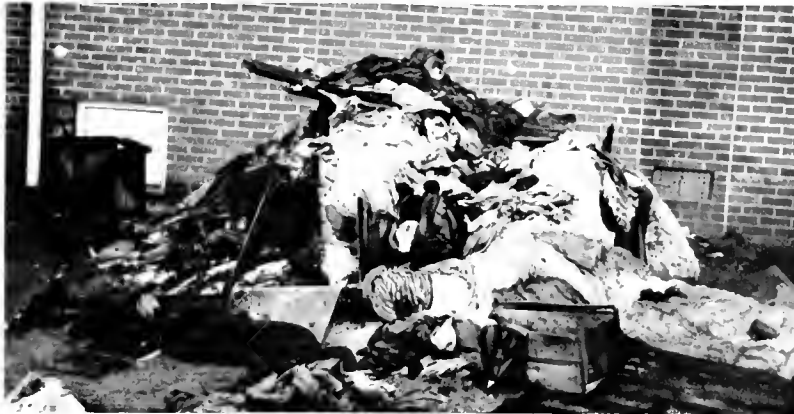
Pictured above is what was left after a fire burned Apartment 3 in the New Complex in late November.
