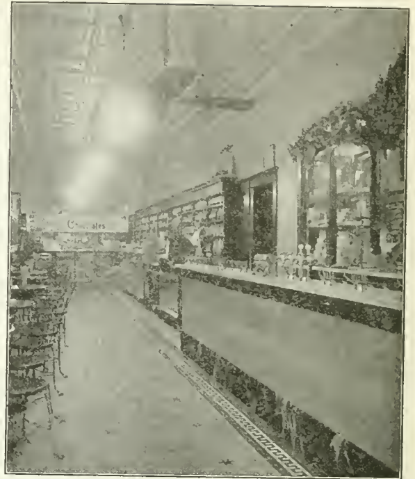
Fig. 4—A Drug Store Using Mazda Lamps equipped with Opalescent Glass Enclosing Globes and Flat Steel Reflectors.
