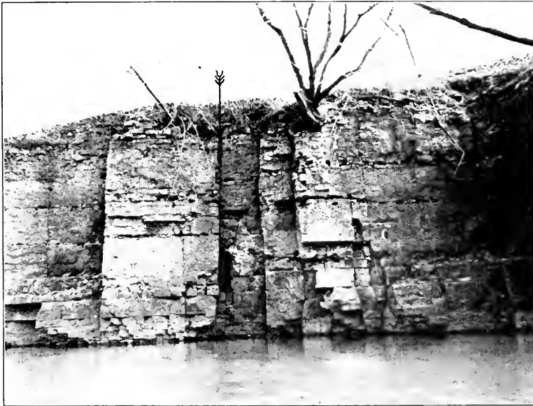
B. Fault in the Wall of Sugar Creek Gorge. The fault fracture cuts the large rectangular opening. The block on the right is a foot above that on the left.
