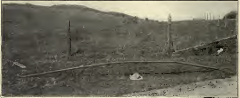
FIG. 457.—A water-pipe buckled out of the ground by the earthquake. Alpine road, Portola Valley, Cal. (Photo. by Dudley.)
