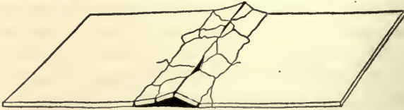
FIG. 69.—A cement walk broken under expansion by sun-heat.
