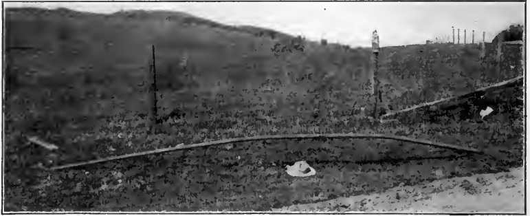
FIG. 457.—A water-pipe buckled out of the ground by the earthquake. Alpine road, Portola Valley, Cal. (Photo. by Dudley.)
