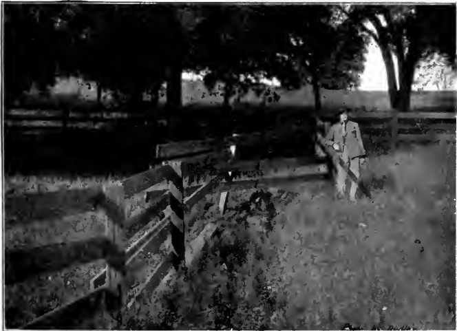
FIG. 456.—A broken (now mended) and offset fence. That in the foreground was formerly in line with the single length directly behind the man.
