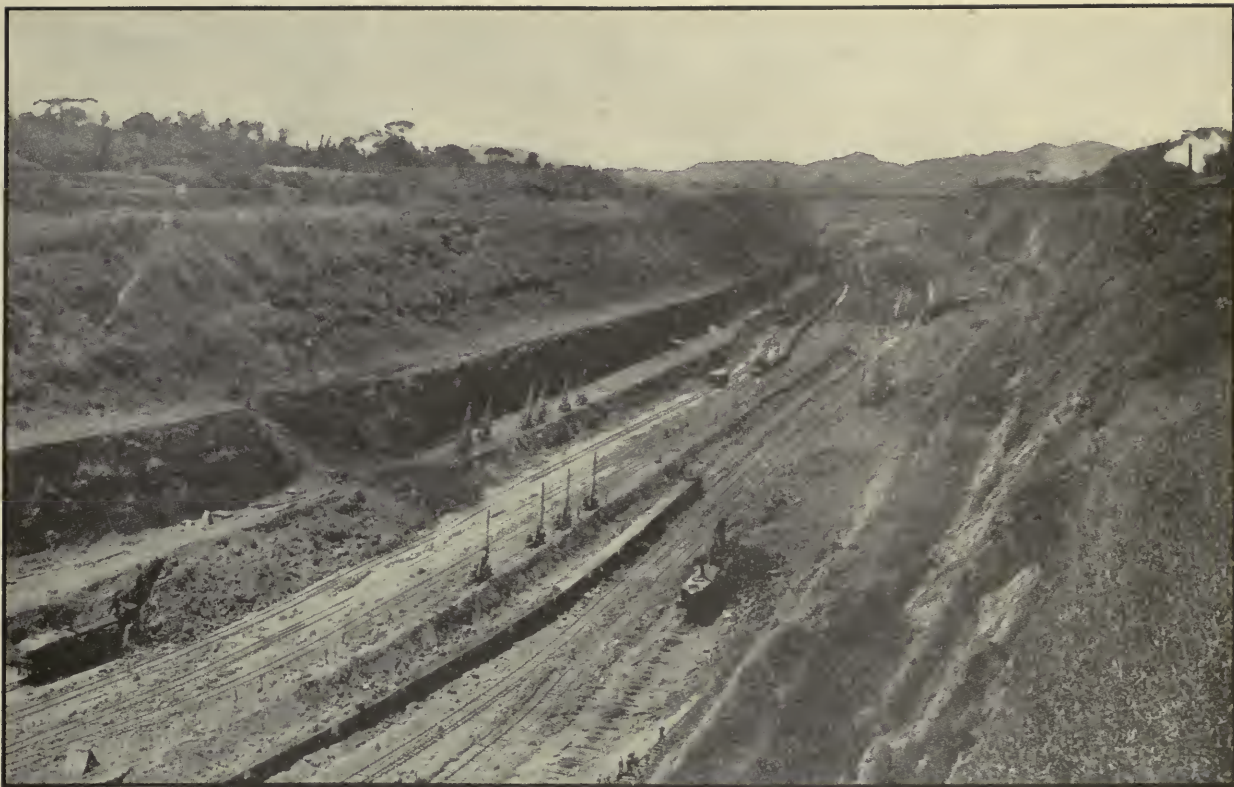
Culebra Cut, Looking North from a Point South of Contractor's Hill, Showing Quiescent State of the Great Cucaracha Slide on Right Bank. Photographed May, 1912.
