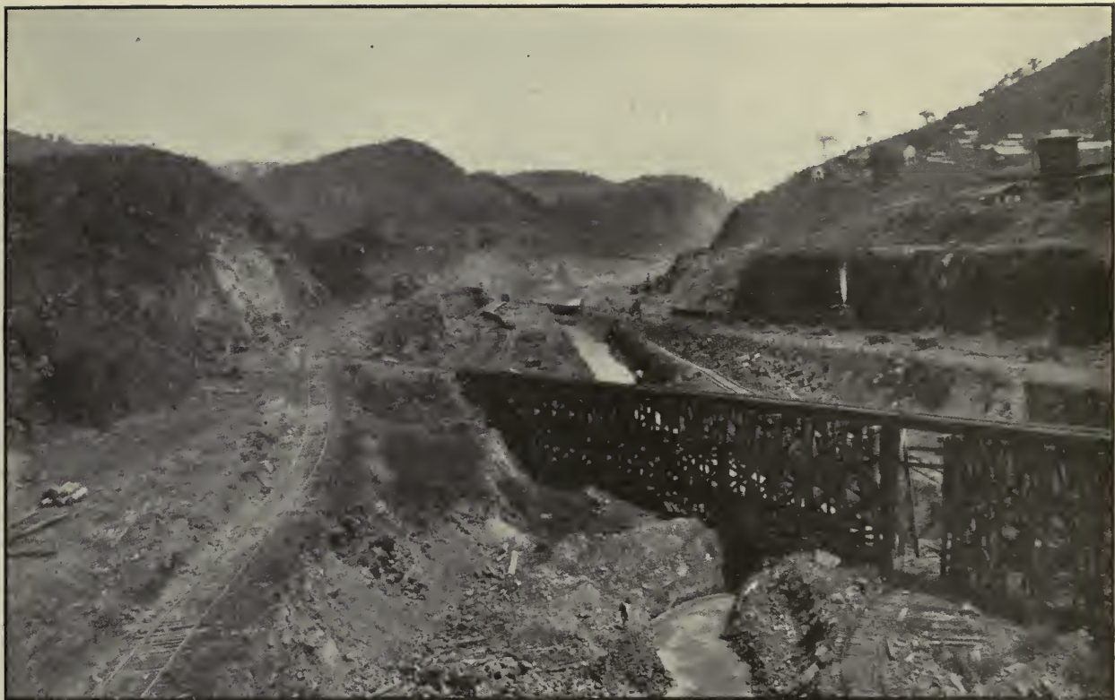
Culebra Cut Looking North from Bridge 57½, Near Paraiso. The Train on the Left, Just Beyond the Trestle Bridge, Is on the Completed Bottom of the Canal, Elevation +40. Photographed June, 1912.
