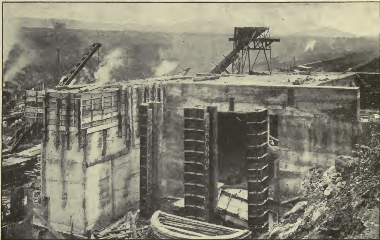
Miraflores Upper Locks, Showing Stoney Gate Valve Frames in Position in South End of West Wall. Photographed November 8, 1911.
