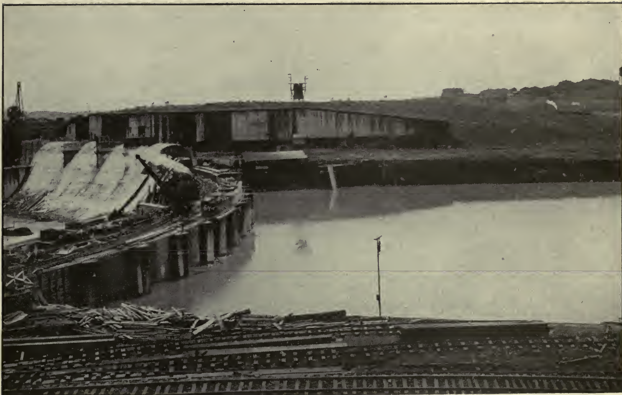
Gatun Spillway Looking East Toward Locks, Showing Up and Down Stream Faces of Ogee Dam, June 6, 1912. The Spillway Will Be Used to Regulate the Water Level of Gatun Lake.
