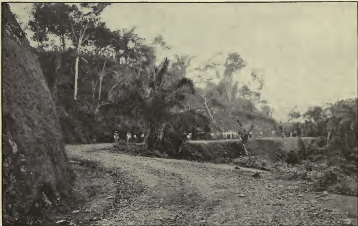
Empire-Chorrera 16-Foot Macadam Road Under Construction with Zone Prison Labor, as It Appeared August 29, 1912.
