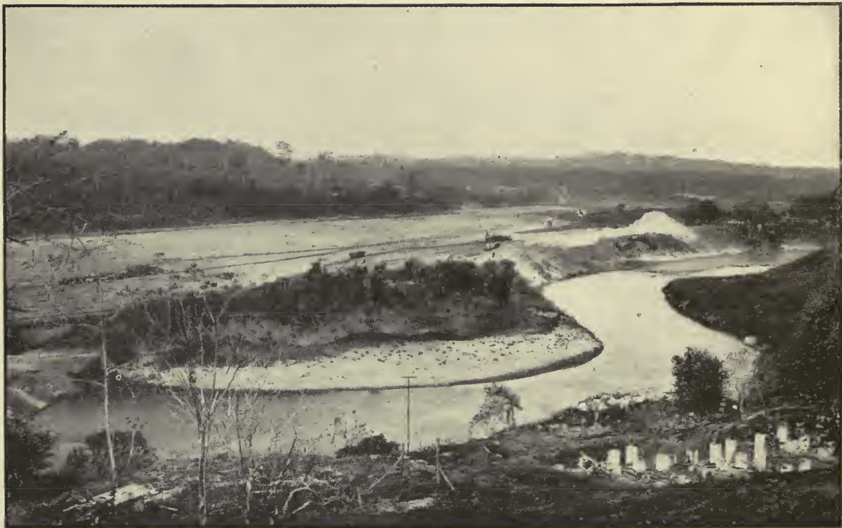
Channel Excavated at San Pablo During Dry Season, 1912. This Channel Is Completed and Is 800 Feet Wide, With Bottom Elevation at +40.
