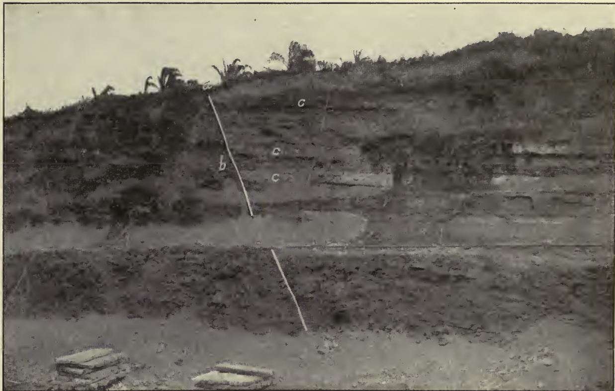
"A" Fault Plane. "B" Crushed and Sheared Zone of Rock. "C" Stronger Rocks, Beds of Limy Sandstone. This Fault Was the Chief Cause of the Big Slide on the West (Opposite) Side of the Canal Near Lirio.
