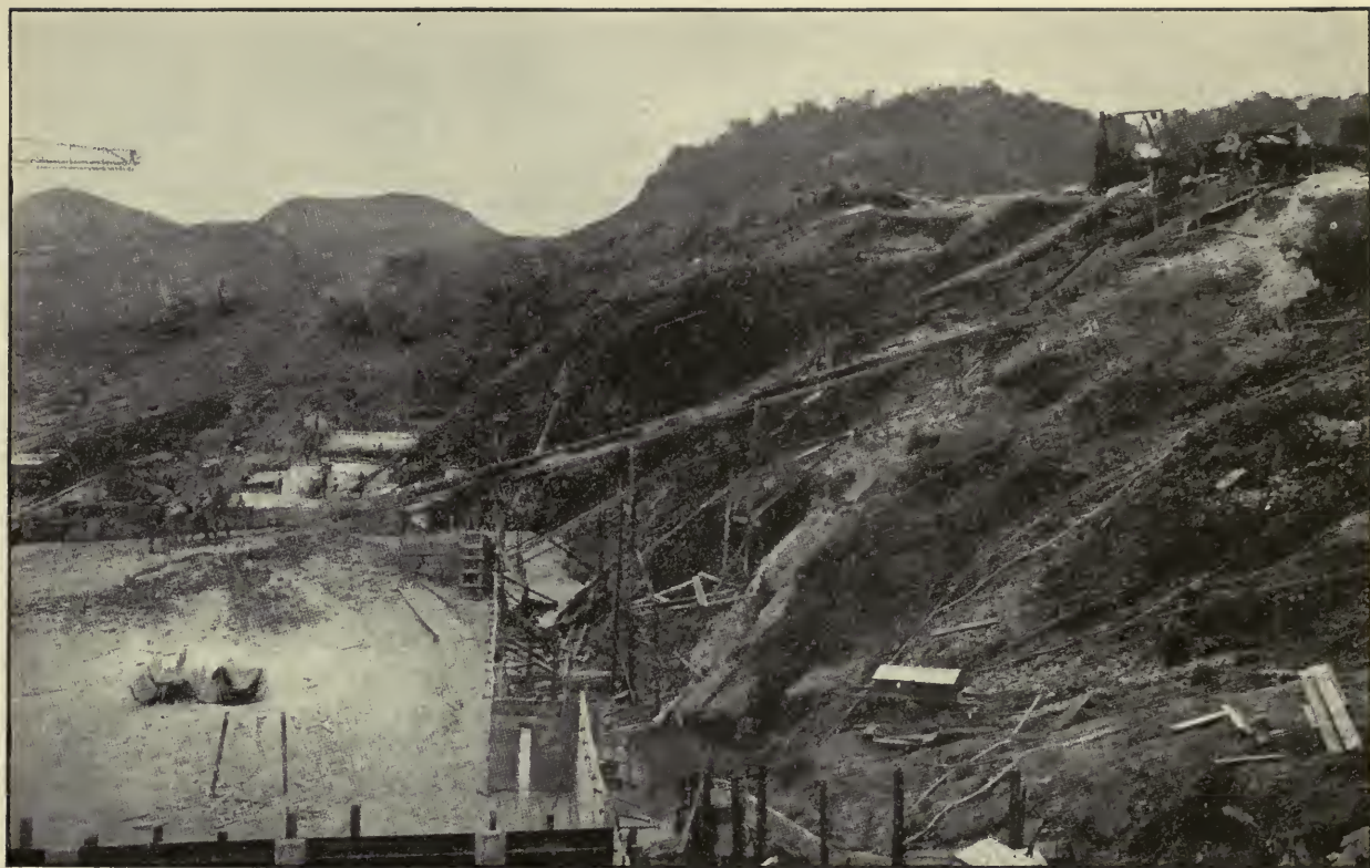
Miraflores Lower Locks. Slide Back of West Wall, Looking South, as It Appeared March 21, 1912.
