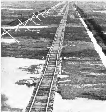
FIG. 3—Telephone line on temporary tripods and new track in undeveloped country, Hudson Bay Railway. (Canadian National Railways.)
