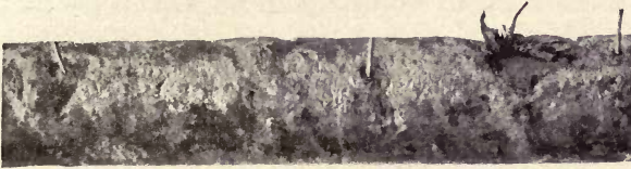
Another View of Burlap-Covered Mannesmann (Steel) Pipe Badly Damaged by Rust
