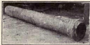
Cast Iron Gas Pipe 83 Years in Service in Baltimore, Md.
