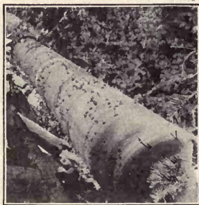
Steel Pipe Line in Oregon Abandoned After Less than 15 Years' Service
