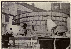
Taking Down Old Cast Iron Tank in 1914—After More Than 100 Years Service
