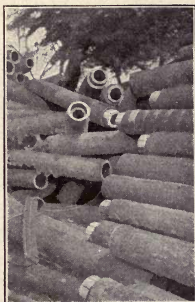
Wood Pipe, Conway, Arkansas, Replaced After Four Years by Cast Iron Pipe
