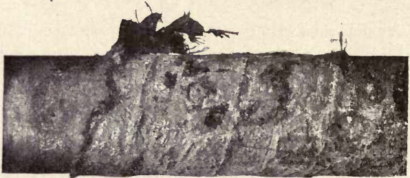
Mannesmann (Steel) Pipe, Burlap Covered, Replaced After 11 Months' Service. Close Alongside is a Line of Cast Iron Pipe in Service 13 Years Without Apparent Defect.
