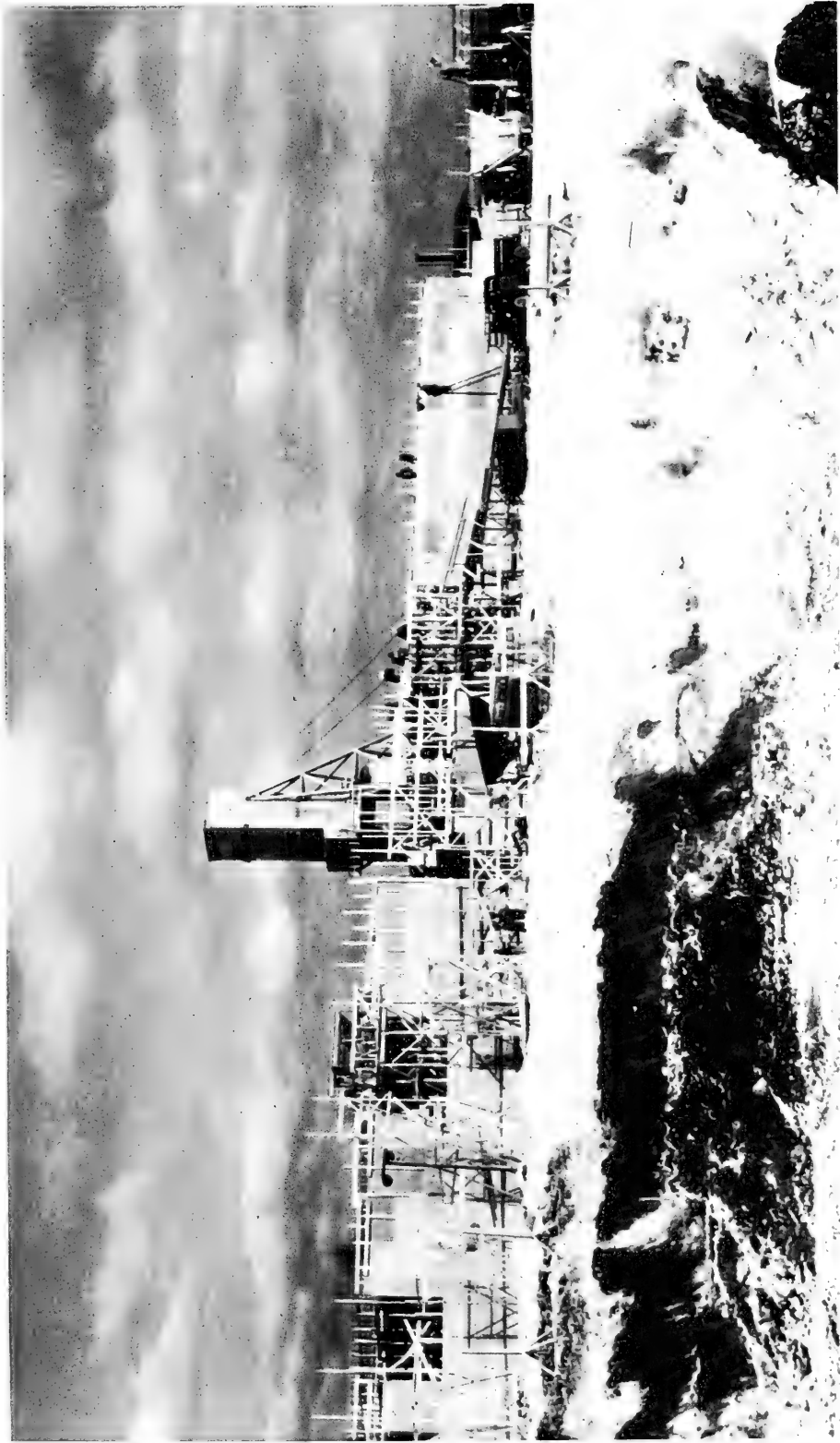
Fig. 9 — NORTH POLAR REGION: MINING. Temporary headframe housing No. 1 shaft and part of concentrator foundations at the Thompson, Manitoba, plant. The plant will process nickelferous ores. (Photograph courtesy of International Nickel Company.)
