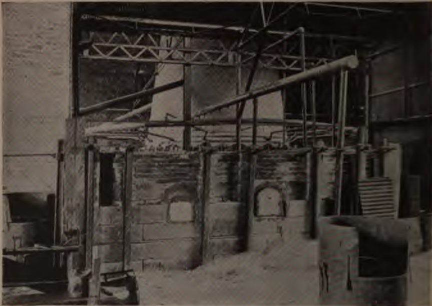
TANK FURNACE USED IN THE MANUFACTURE OF LAMP CHIMNEYS AT JEANNETTE, PA.
