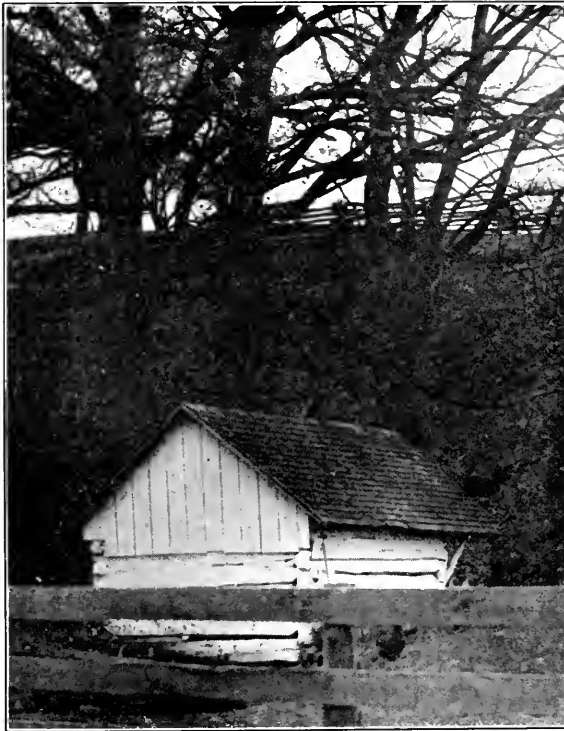
SAWED SHINGLES AND A FEW BOARDS ARE USED IN LENGTHENING THE YEARS OF SERVICE OF THIS ROUGH-HEWN LOG SPRING HOUSE.
