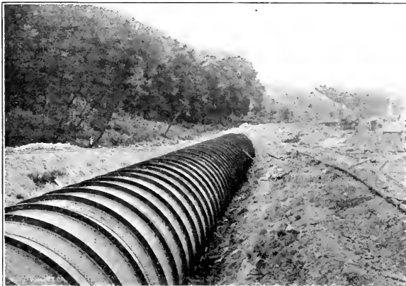
EIGHTEEN-FOOT CONDUIT, ONTARIO POWER COMPANY, NIAGARA FALLS, ONTARIO.
