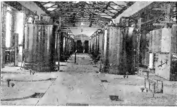
TRANSFORMER PLANT OF NIAGARA FALLS POWER COMPANY.
