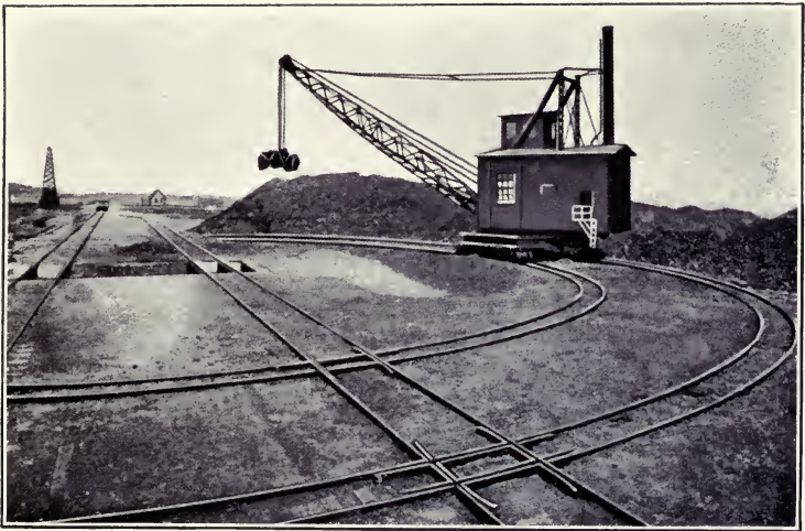
STEAM CRANE FOR CIRCULAR COAL STORAGE SYSTEM (20 ft. gauge, 80 ft. radius, 2 ton bucket, 80,000 tons storage capacity).
