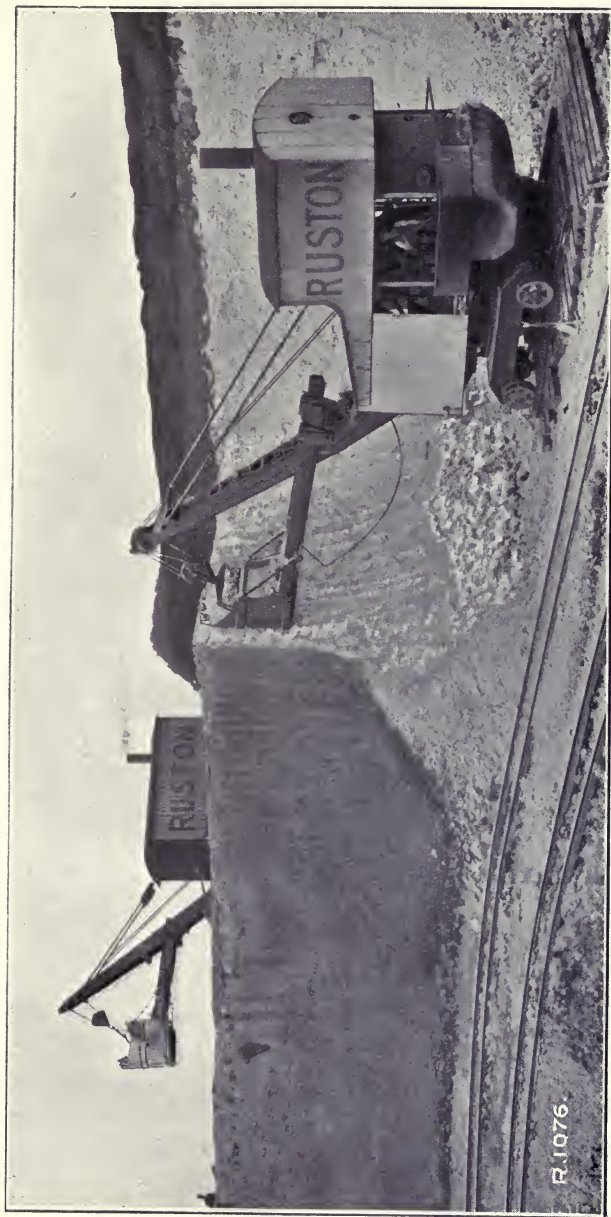
Showing the usefulness of the CRANE NAVVY in quarry work. The machine at the top is removing the top soil or overburden, and the machine in the bottom is excavating the mineral, which in this case is chalk for making cement.
