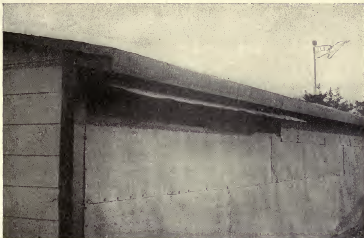
• FIG. 67.—An efficient rear ventilator for summer use. It allows the air to enter the back of the house, and circulate between the sheathing and the roof, cooling the roosting quarters on summer nights. This is most valuable for shed-roofed houses that are covered with paper. Cornell University was the first Experiment Station to recommend back ventilation for the poultry house.
