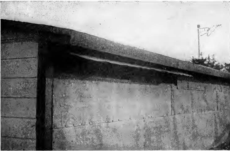
♦ FIG. 67.—An efficient rear ventilator for summer use. It allows the air to enter the back of the house, and circulate between the sheathing and the roof, cooling the roosting quarters on summer nights. This is most valuable for shed-roofed houses that are covered with paper. Cornell University was the first Experiment Station to recommend back ventilation for the poultry house.
