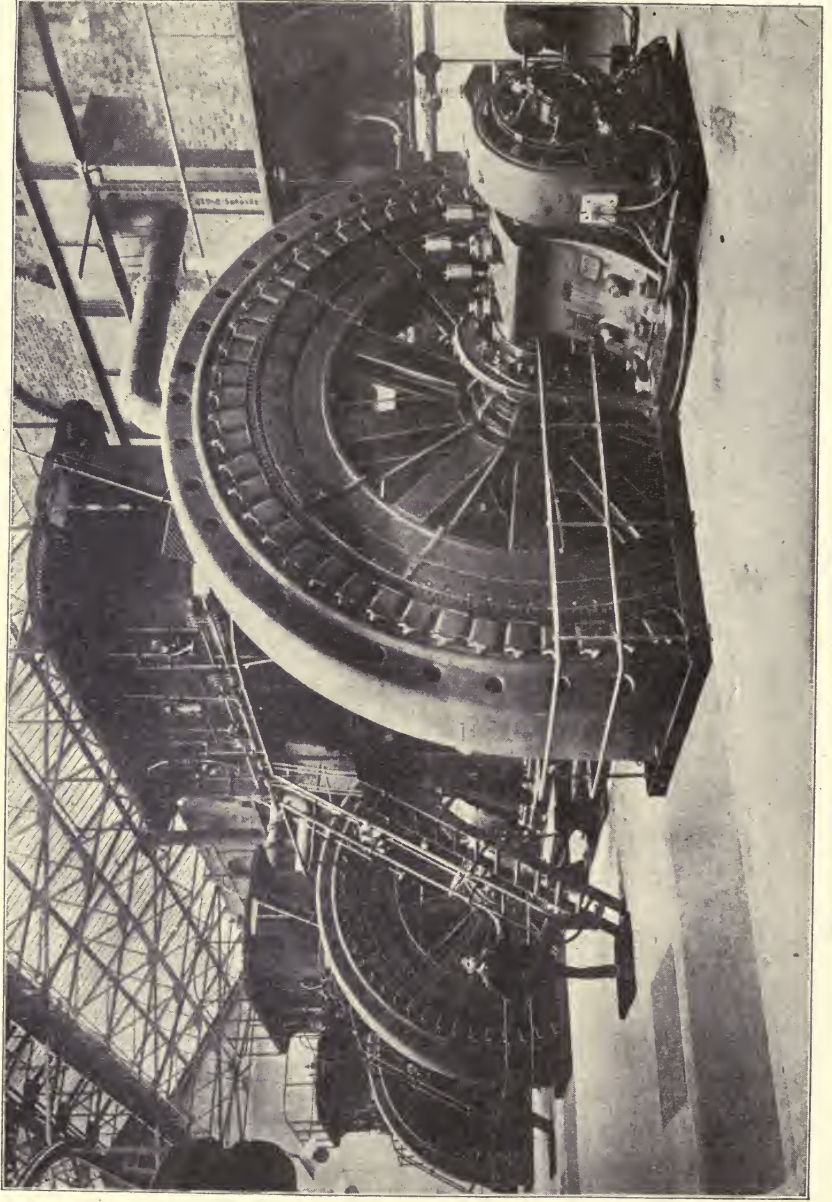
WESTINGHOUSE TWO-PHASE GENERATORS, DIRECT-CONNECTED. Metropolitan Electric Supply Co., Ltd., London, England.
