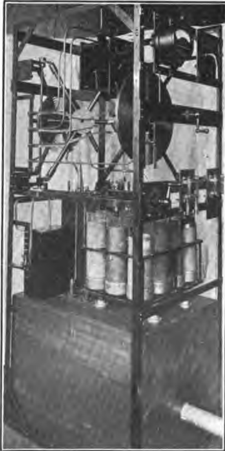
Fig. 146a—3 Kilowatt Non-Synchronous land station type of transmitter (American Marconi Company).
