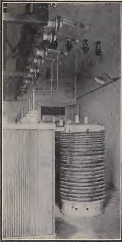
Fig. 307—Bank of High Voltage Transformers at Carnarvon Station.
