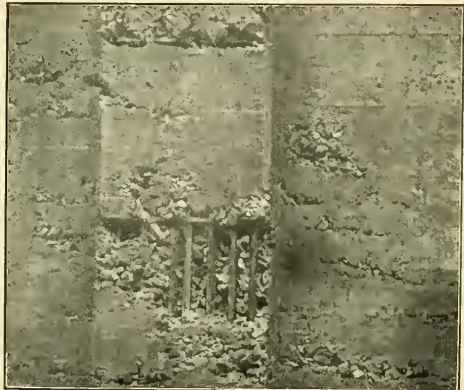
FIG. 3.—CAVITIES IN COLUMN.
