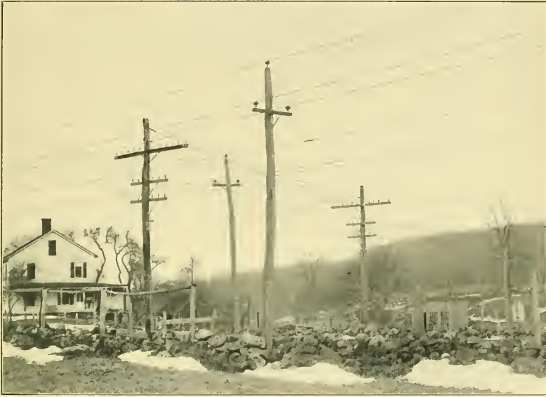
FIG. 1.—WIRE GRIDIRON UNDER 33 000-VOLT TRANSMISSION LINE.
