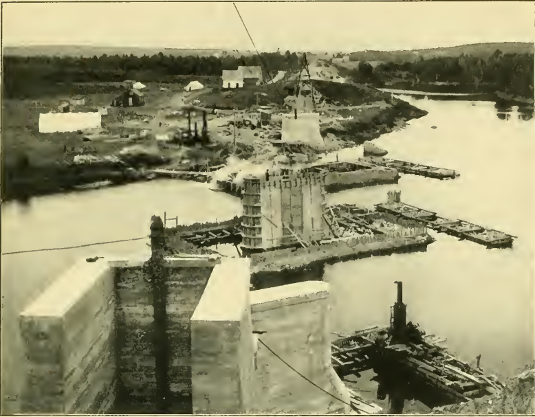
FIG. 1.—GENERAL VIEW, LOOKING SOUTH. NORTH ABUTMENT AND PIERS 1 AND 4 FINISHED. PIER 2 NEARLY COMPLETE, AND PIER 4 BEING EXCAVATED.
