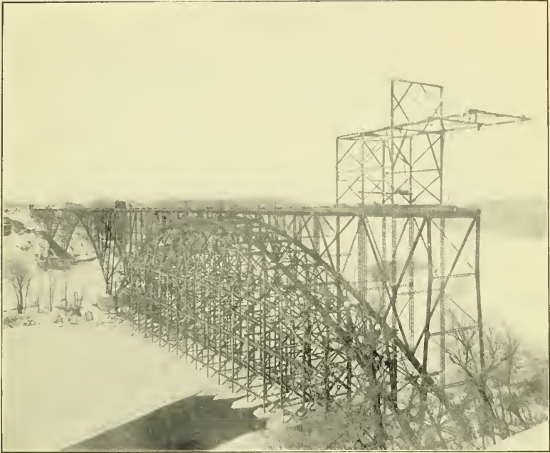
FIG. 1.—THE ERECTION OF THE LAKE STREET BRIDGE, OVER THE MISSISSIPPI RIVER, AT MINNEAPOLIS.
