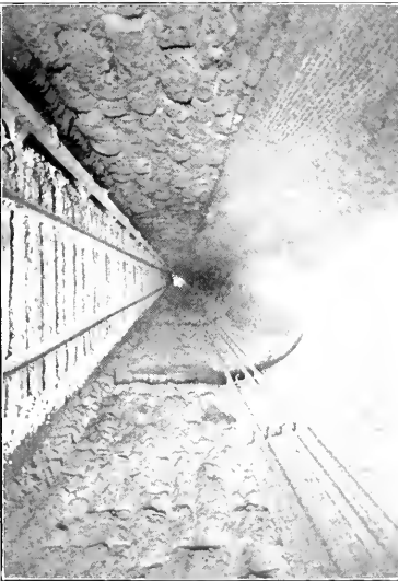
FIG. 4.—STREET TRANSMISSION LINE IN BRICK TUNNEL.
