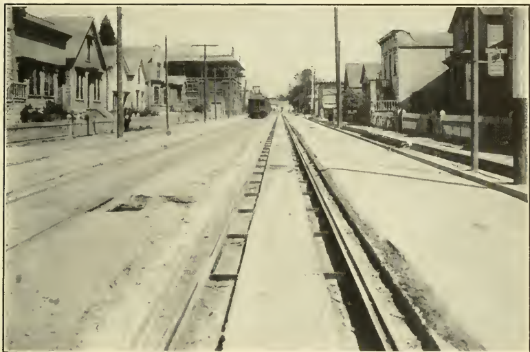
FIG. 1.—ASPHALT PAVING, TWENTY-SECOND STREET, OAKLAND, CAL. GIRDER-RAILS, STEEL TIE-PLATES, WOODEN TIES, CONCRETE TO BASE OF TIE, BASALT BLOCK LINERS ON 1\frac{1}{2} -IN. SAND CUSHION.
