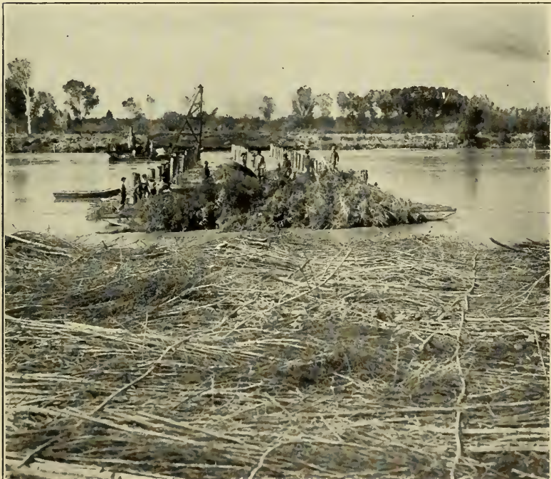
FIG. 2.—EDINGER DAM, NOVEMBER 8TH, 1905. BRUSH AND WIRE MAT IN FOREGROUND, READY TO BE PLACED.
