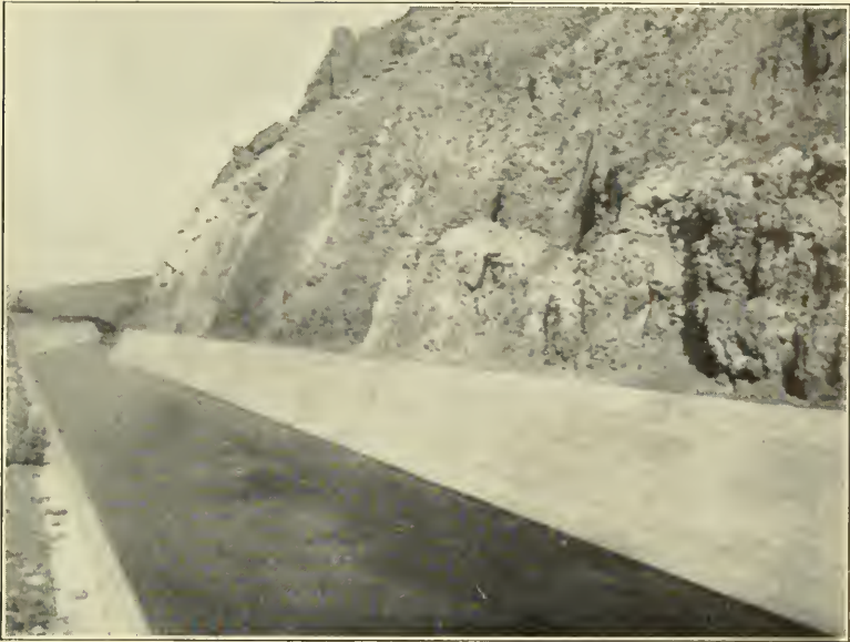
FIG. 1.—MAIN CANAL, TRUCKEE PROJECT, CONCRETE LINED.
