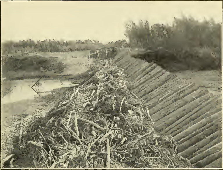
FIG. 1.—TYPICAL ABATIS WORK ON LEVEES OF YUMA PROJECT, U. S. RECLAMATION SERVICE.
