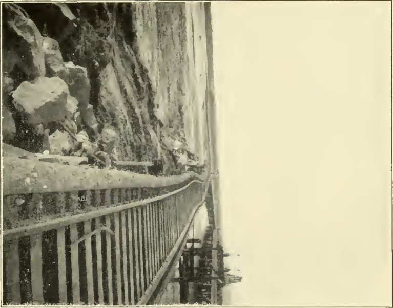
FIG. 1.—KINK IN LOWER TRESTLE CAUSED BY DRIFT BREACHING AND TAKING OUT FOUR BENTS OF UPPER TRESTLE.
