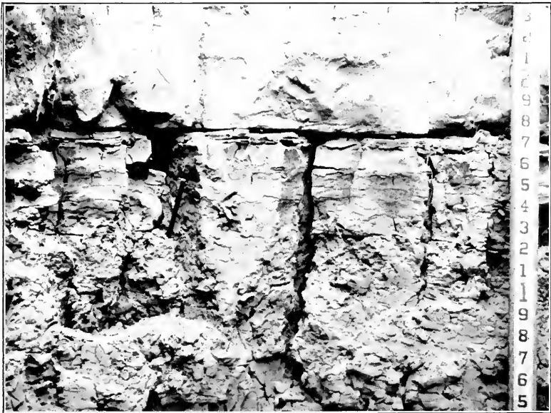
FIG. 2.—TYPICAL SUBSURFACE OF CRACKED ADOBE MATERIAL. THE BOTTOM OF THE ROD IS 5.3 FEET BELOW THE SURFACE.
