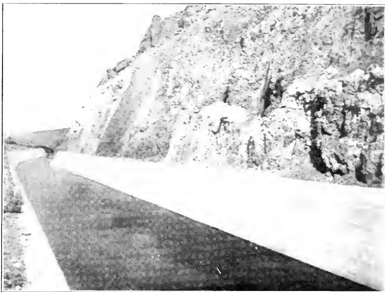
FIG. 1.—MAIN CANAL, TRUCKEE PROJECT, CONCRETE LINED.
