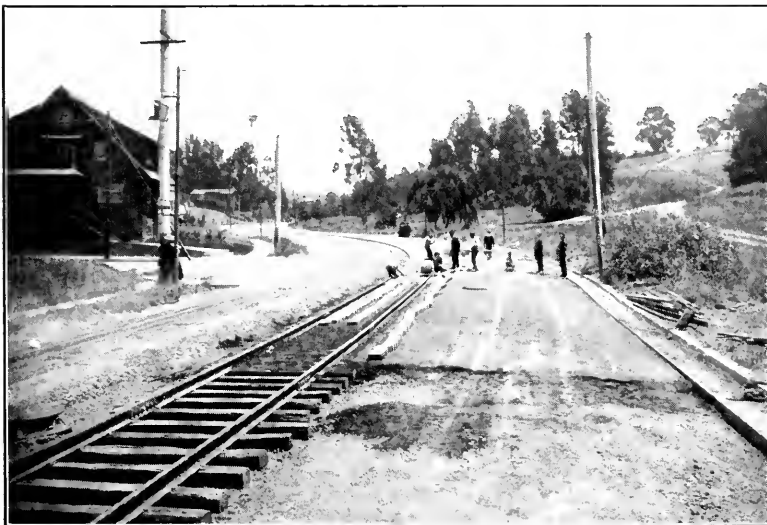
FIG. 2.—ASPHALT PAVING, FOURTH AVENUE, OAKLAND, CAL. VITRIFIED BRICK LINERS. ASPHALTIC CONCRETE BETWEEN TIES, INSTEAD OF HYDRAULIC CONCRETE.
