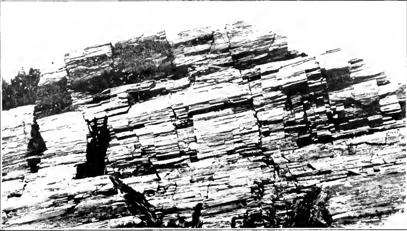
FIG. 3. JOINT DISINTEGRATION, PROUT'S NECK, MAINE
