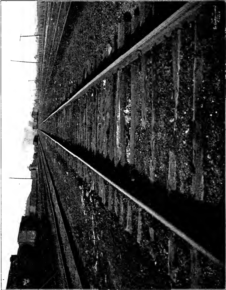
Rail-Cutting on Track Not Provided with Tie-Plates.
