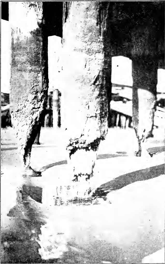
FIG. 26.—TIMBER PILES DESTROYED BY LIMNORIA IN OAKLAND HARBOR, CALIFORNIA.
