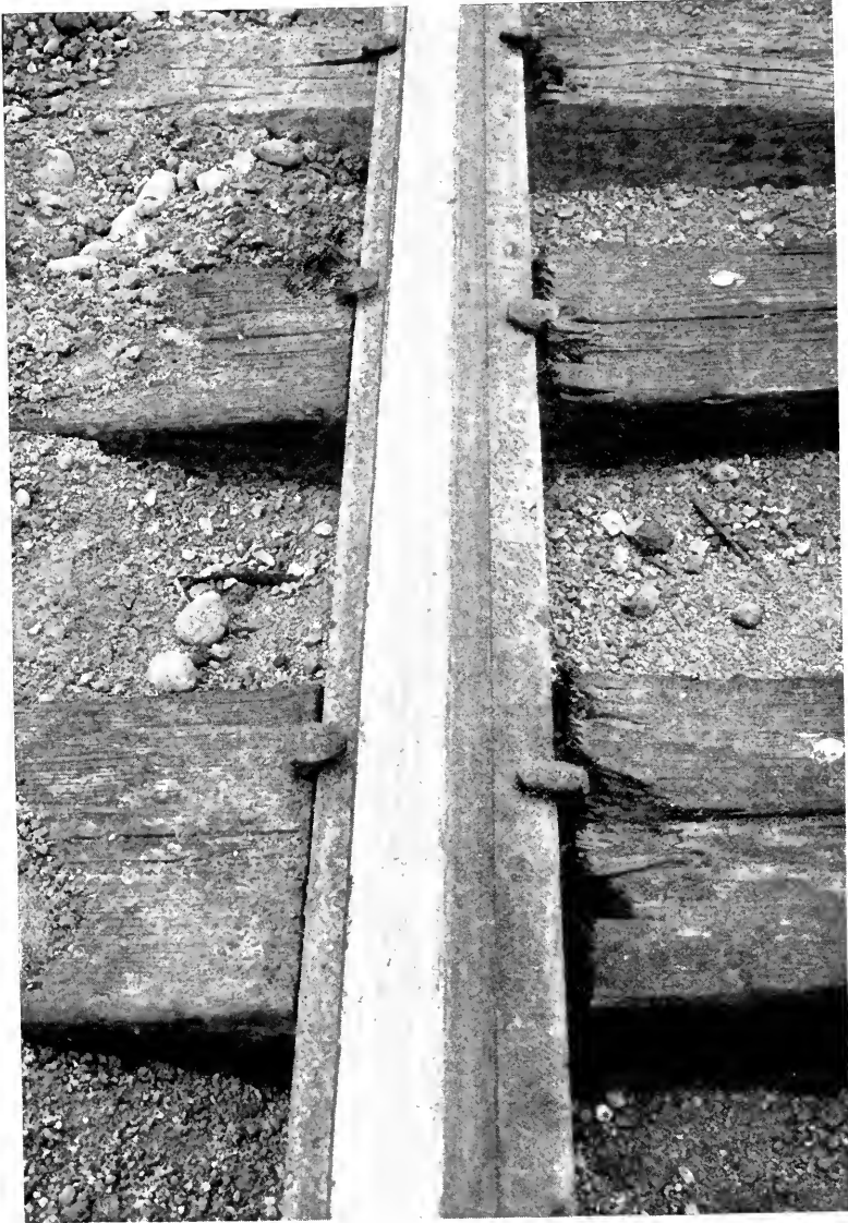
View showing injury to ties by rail cutting and spike driving. View 22, Arkansas River Division, 1910 treated ties, with cut spikes without plates. Note especially ruination of ties in three years from this cause.
