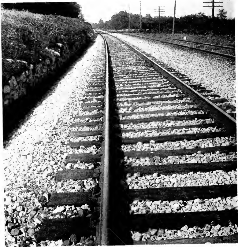
Betts anti-creeper tie plate, on curve just west of Turner Station.
