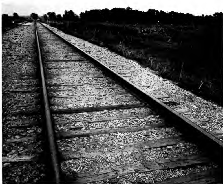
View 12; 1912 screw spikes on ties in quarter and centers.
