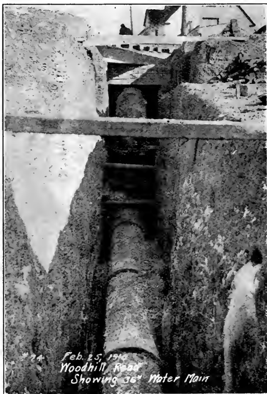
FIG. 31—36-INCH WATER MAIN AT WOODHILL ROAD.
