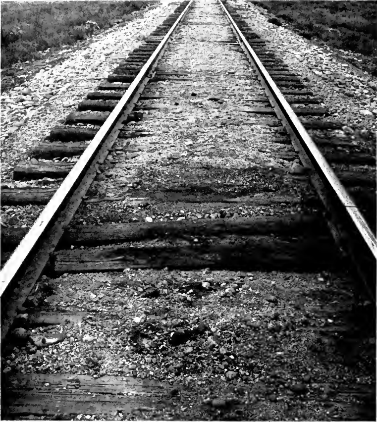
View 2, Arkansas River Division. Cut-spike track without tie plates or rail anchors. Note the damage to tie from rail cutting and condition of track account skewing of tie.
