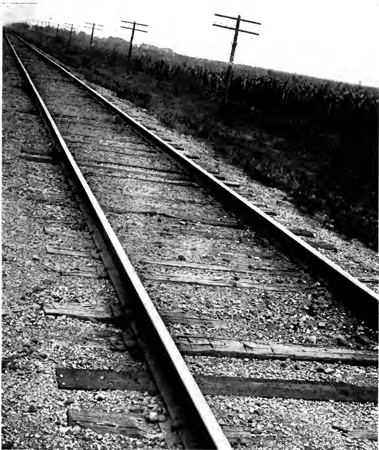
View 23, Illinois Division, showing cut-spike track with tie plates and rail anchors.
