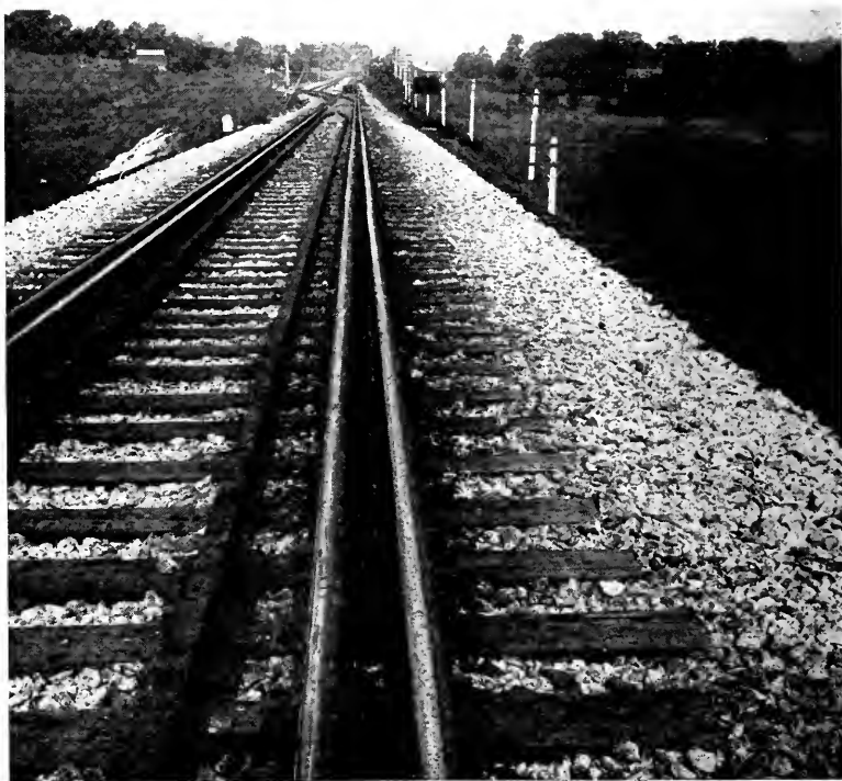
View 23, Missouri Division. Gauntlet track with screw spikes, standard construction screw spikes.
