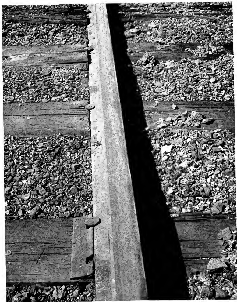
View showing injury to ties by rail cutting and spike driving. View 21, Colorado Division, showing ties with and without tie plates.
