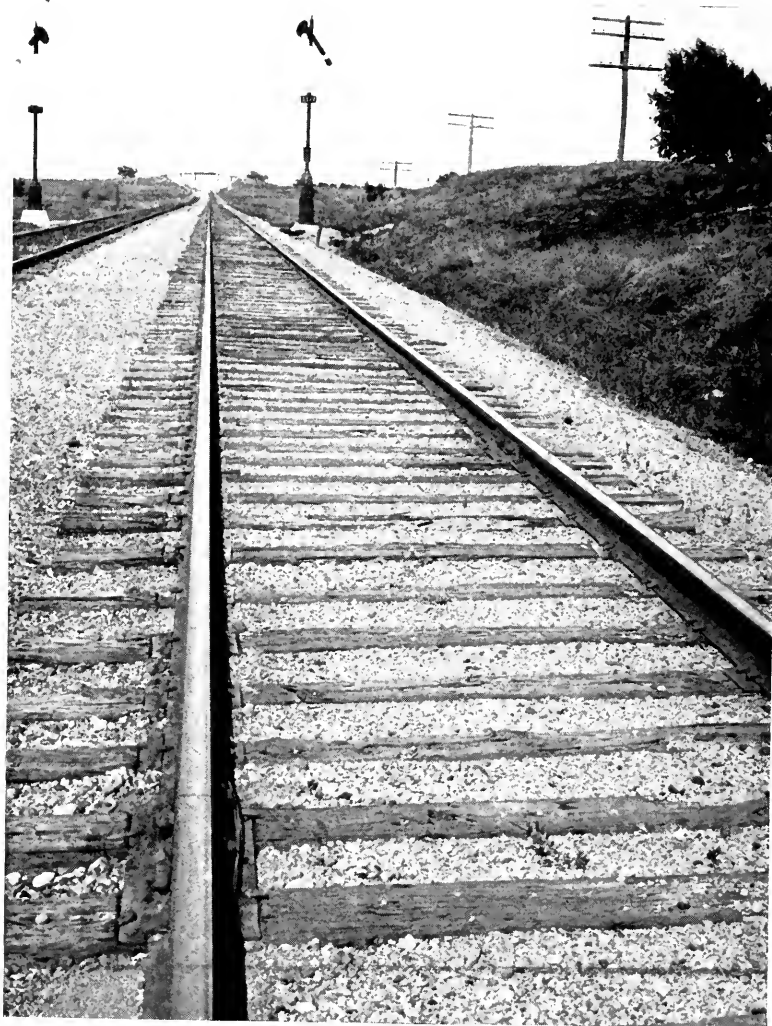
View showing injury to ties by rail cutting and spike driving. View 3. Missouri Division. Cut-spike track with tie plates, where zinc ties used same as in View 2. These ties being laid out of face when track was constructed and right at end of the tie shown in No. 2. Observation on ground would indicate would get at least four years more service from the ties than those without plates, and if ties had been high-class creosoted ties in first instance, this would be increased.
