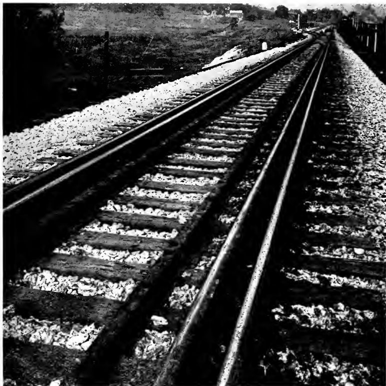
View 24. Missouri Division. Gauntlet track, with screw spikes; standard construction screw spikes.
