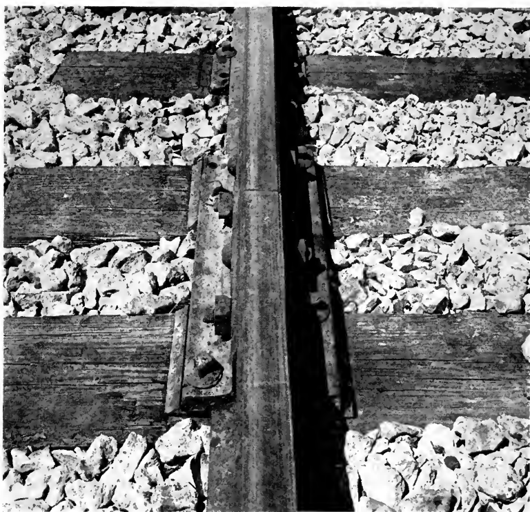
No. 3. View 23. Western Division. Beddoe Joint with screw spikes. Roadmaster claims better service with screw spikes than Weber.
