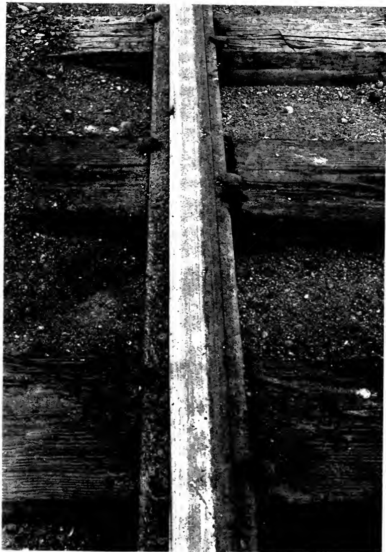
View showing injury to ties by rail cutting and spike driving. View 3, Arkansas River Division. Same as View 22.
