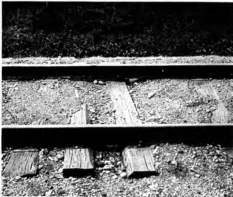
View 21, Illinois Division. Screw spike; joint ties inserted without tie plates. Note skewing, which is approximately 4 in. and is average of the lot.
