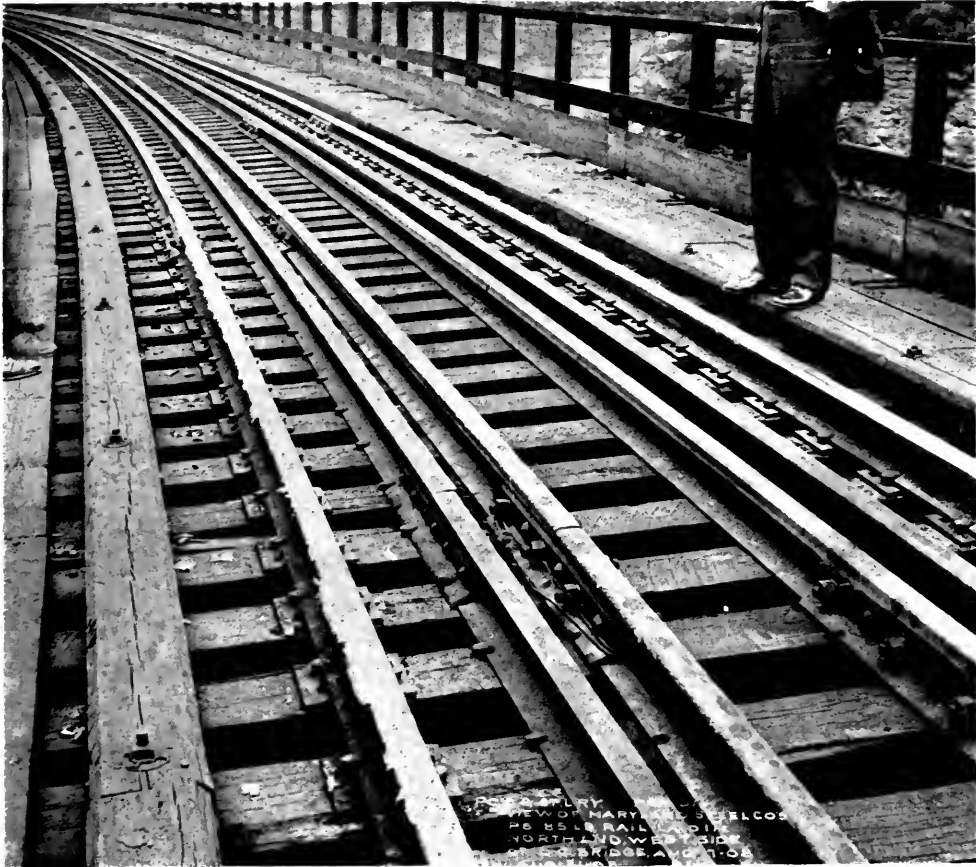
FIG. 84. FLOW OF METAL, MARYLAND RAIL. OHIO CONNECTING BRIDGE.
