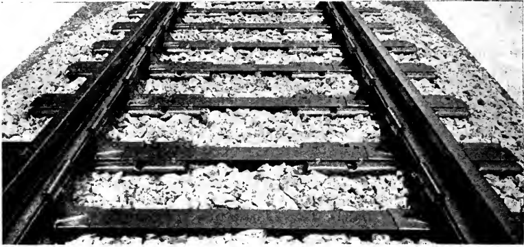
FIG. 6. LONGITUDINAL VIEW OF THE NEW DESIGN MORGAN TIE IN SERVICE AT ATGLEN ON THE PENNSYLVANIA RAILROAD.
