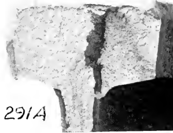
FIG. 291A. SHOWING SPLIT IN CRUSHED HEAD OF RAIL 291.
