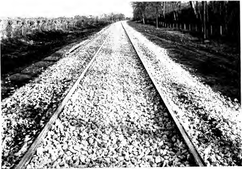
FIG. 22. TRACK AFTER BALLAST HAS BEEN DROPPED AND BALLAST SPREADER AND FORMER HAS GONE OVER IT.
