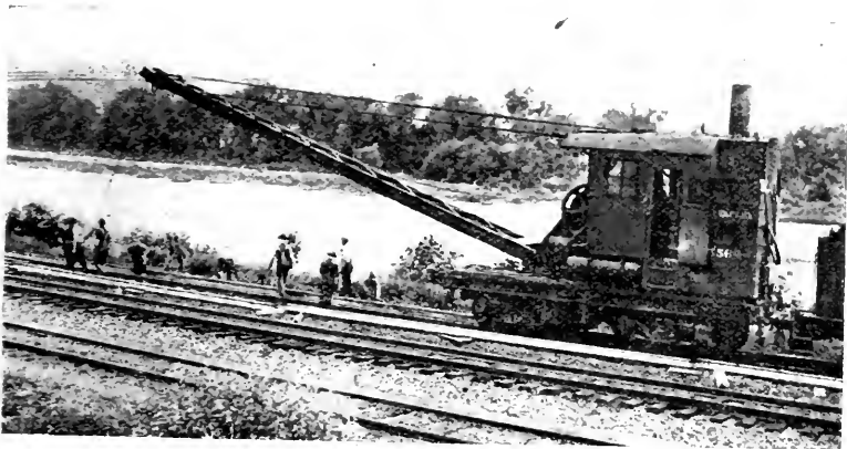
FIG. 6—DRILLING OUTFIT MOVING AHEAD, AFTER DRILLING FOUR HOLES, OR TWO JOINTS, TO NEXT TWO JOINTS.
