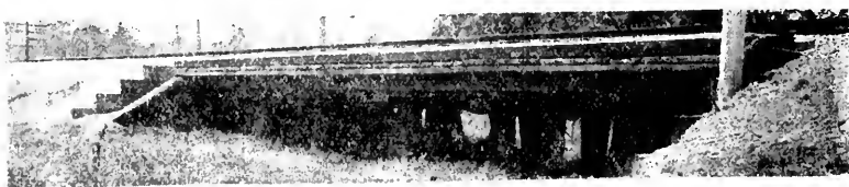
Picture 80. Trestle 488-G, Southern Pacific, west of Stoneman, between Los Angeles and Colton, 45 feet, constructed of creosoted Douglas fir in 1901, with 12x12 creosoted stringers covered with 3x12-14 creosoted fir plank for ballast. These planks were added 1903, three helper bents added 1925, account heavy traffic and are untreated material. New dump bent put in in 1927. Original creosoted timbers in good condition. Photographed August 9, 1928.
