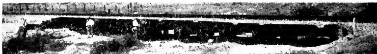
Picture 98. Trestle 451-B, Southern Pacific, east of Saugus. Length, 90 feet, constructed of creosoted Douglas fir 1897. Stringers are 12 x 12 solid type construction, seven bents of four piles each. Five of the piling have been renewed. Helpers have been placed in the bents to take care of heavy traffic. Four caps replaced account of crushing. Photographed August 10, 1928.
