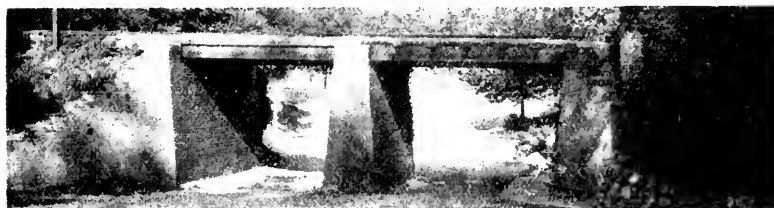
Picture 90. Bridge 513-J, Southern Pacific, Covina Branch, Genesha Park, Pomona, Calif. One 19-foot span contains 29 7 x 16—20's and one 17-foot span contains 21 7 x 16—18 creosoted fir stringers placed in 1896. All in sound condition. Photographed August 9, 1928.
