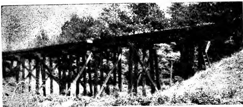
No. 10. C. R. I. & P. bridge 905, between Haskell and Eldorado, Ark. Constructed 1914. Six stringers per panel, creosoted Douglas fir in original bridge. Two additional stringers, creosoted pine, added later. Photographed May 24, 1928.
