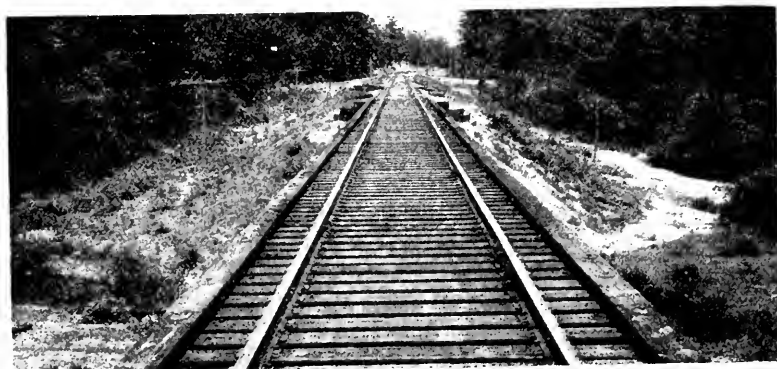
No. 13. C. R. I. & P. bridge 905, between Haskell and Eldorado, Ark., constructed 1914. Four-inch guard rails bolted to ties. Photographed May 24, 1928.
