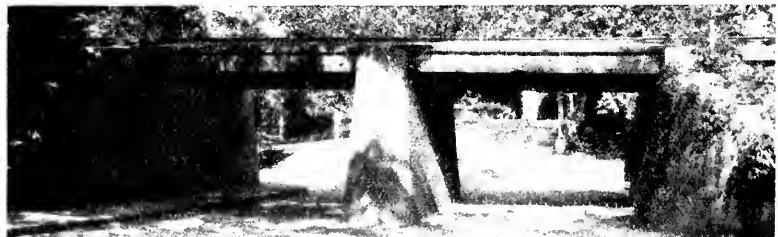
Picture 88. Bridge 513-K. Southern Pacific, on the Covina Branch, Genesha Park, Pomona, Calif. Constructed 1896. Creosoted Douglas fir stringers resting on brick piers. Two 17-foot spans each having 21 7 \times 16 -18's all in absolutely sound condition. Ends of stringers bear on creosoted 6 \times 12 's which in turn rest on the brick. Photographed August 9, 1928.
