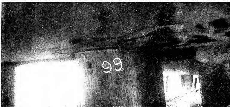
Picture 99. Trestle 451-B, Southern Pacific, east of Saugus. Creosoted Douglas fir, constructed 1897. Close-up of cap showing crushing over pile. These were originally four-pile bents. Helpers placed in recent years account heavy traffic. Photographed August 10, 1928.
