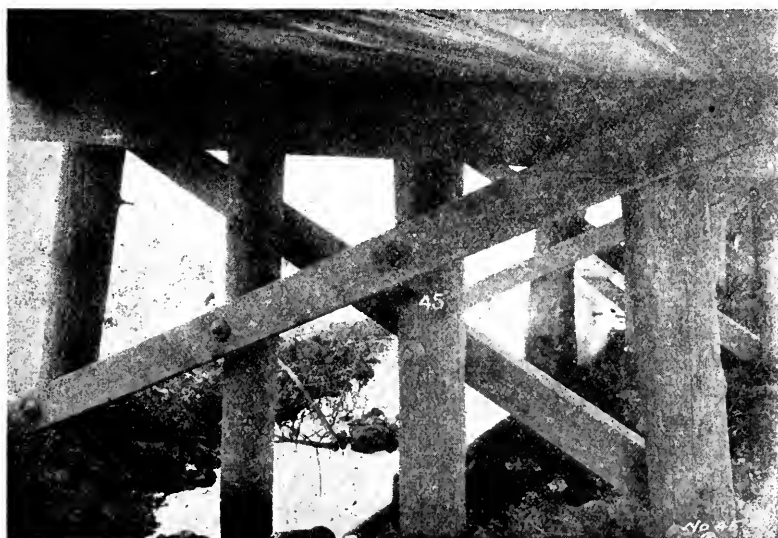
Picture 45. Trestle 45-E, Calistoga Line, Southern Pacific, 195 feet, CSB-4, built 1900 of creosoted Douglas fir. Close-up of 4-pile bent. Note excellent condition after 28 years' service. Photographed August 6, 1928.
