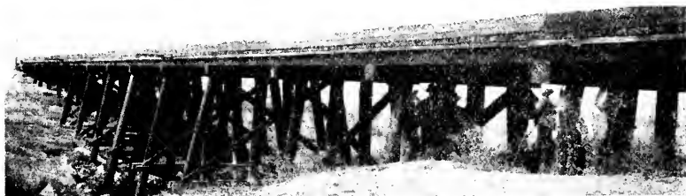
Picture 68. Trestle 60-B, Southern Pacific, Oakland to Tracy, 240 feet, CSB-4. Constructed of creosoted Douglas fir 1900. Contains 17 bents, 6 of the bents, 6 piles each, the remainder 4. New caps applied 1927. 12 x 14's laid flat. Some new guard timbers have been applied, replacing original guard timbers broken unloading riprap. Photographed August 7, 1928.
