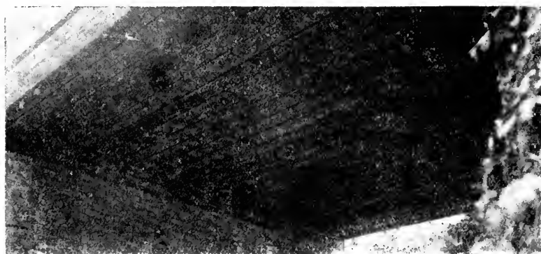
Picture 91. Bridge 513-J, Southern Pacific, Covina Branch, Genesha Park, Pomona, Calif. Close-up of creosoted fir stringers placed in this bridge in 1896, still in excellent condition. This bridge has one 19-foot span with 29 7 x 16—20's and one 17-foot span with 21 7 x 16—18 stringers. Ends of the stringers rest on creosoted 6 x 12's. Photographed August 9, 1928.
