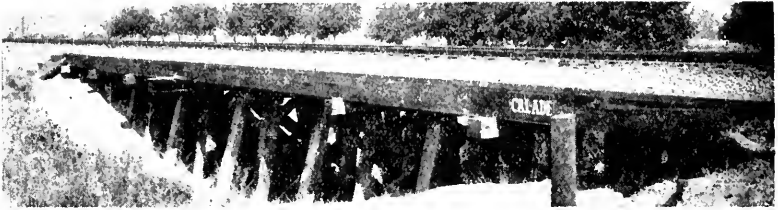
Picture 86. Trestle 507-E. Southern Pacific, east of Walnut. Length, 105 feet. Constructed of creosoted Douglas fir 1901. Eight original bents, four piles to the bent. Helper bents have been added to overcome deflection under heavy power. Four caps have been replaced, two in 1925 and two in 1927. These failed account of crushing over piling. All deck timbers in excellent condition. Photographed August 9, 1928.
