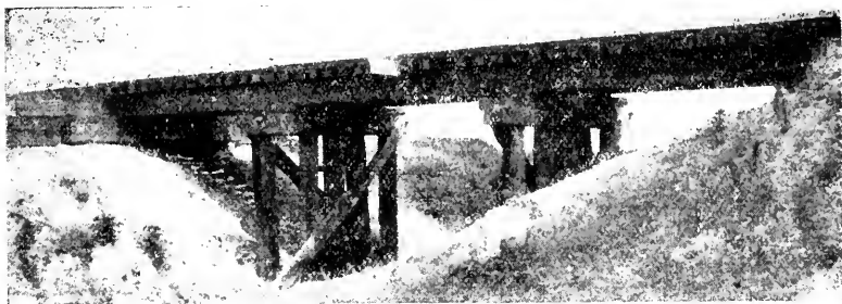
No. 18. C. R. I. & P. bridge 938, Haskell to Eldorado, Ark., constructed 1914. This bridge contains six creosoted Douglas fir stringers per panel, treated with approximately 7\frac{1}{2} pounds of creosote per cubic foot. Two additional creosoted pine stringers added later. Piling, caps and bridge ties creosoted southern yellow pine. Photographed May 24, 1928.
