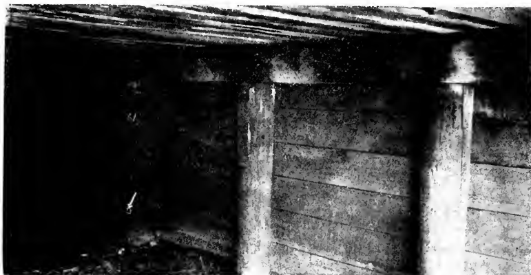
Picture 61. Trestle 9-D, Southern Pacific, at Berkeley, Calif., 12 feet, CSB-4, constructed 1897. Close-up of creosoted piling and bulkhead. Photographed August 7, 1928.
