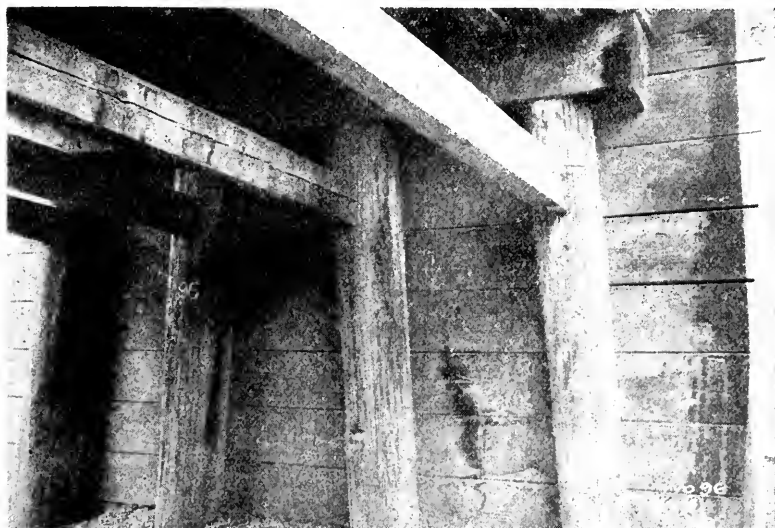
Picture 96. Bridge 460-A, Southern Pacific, east of Sylmar. Length, 15 feet, creosoted Douglas fir, constructed 1897. Close-up of piling which were found, on boring, to be in sound condition. Photographed August 10, 1928.
