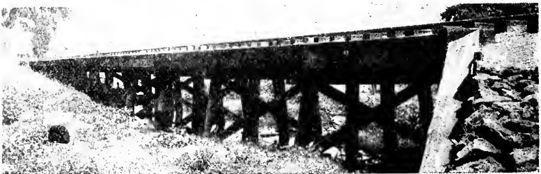
Picture 43-A. Trestle 45-E, Calistoga Line, Southern Pacific, 195 feet, CSB-4, built 1900 of creosoted Douglas fir. No timbers have been renewed in this bridge as yet. Photographed August 6, 1928.
