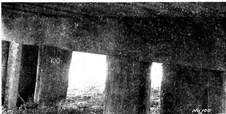
Picture 100. Trestle 451-B, Southern Pacific, east of Saugus. Creosoted Douglas fir, constructed 1897. Close-up of cap showing crushing over pile. These were originally four-pile bents. Helpers placed in recent years account heavy traffic. Photographed August 10, 1928.
