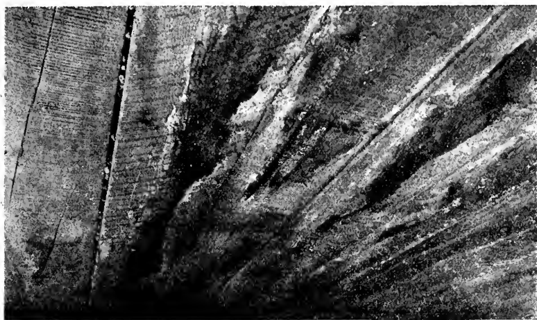
Picture 44. Trestle 45-E, Calistoga Line, Southern Pacific, 195 feet, CSB-4, built 1900 of creosoted Douglas fir. Close-up of creosoted Douglas fir stringers 12 x 12—30. Note slight crushing of cap above piling. Photographed August 6, 1928.
