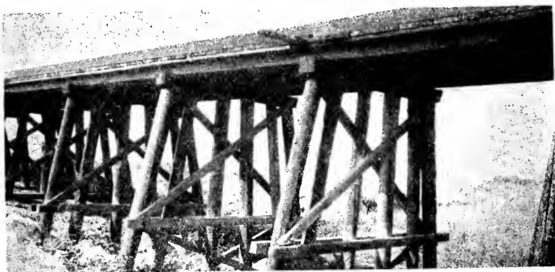
Picture 70. Trestle 60-B, Southern Pacific, Oakland to Tracy. Constructed of creosoted Douglas fir in 1900. Close-up of pile bents. Six bents out of 17 in this trestle are 6-pile bents. The additional piles were added in 1923 to overcome side sway. Photographed August 7, 1928.
