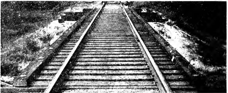
No. 27. C. R. I. & P. bridge 962, Haskell to Eldorado, Ark., constructed 1914. Showing creosoted bridge ties and four-inch guard rails. Ties spaced with four-inch creosoted spacing blocks. Photographed May 24, 1928.
