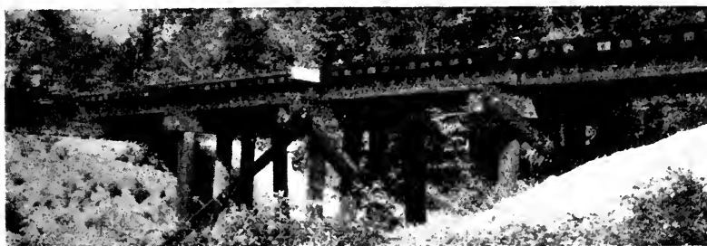
No. 24. C. R. I. & P. bridge 962, Haskell to Eldorado, Ark., constructed 1914. Six creosoted Douglas fir stringers per panel, treated with approximately 7\frac{1}{2} pounds creosote per cubic foot. Two outside stringers, creosoted southern pine applied later. Bridge ties, guard rails, caps and piling all of creosoted southern pine. All in excellent condition and apparently good for many years additional service. Sway braces zinc chloride treated and show decay wherever they come in contact with the ground. Photographed May 24, 1928.
