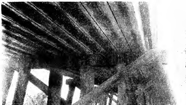
No. 69. Trestle 60-B, Southern Pacific, Oakland to Tracy. Close-up of 6-pile bents. The two outside piles were added in 1923, to eliminate side sway. All of the original 12 x 12 stringers in this bridge still in place. Upon boring into creosoted Douglas fir stringers, some were found with very shallow penetration of creosote, but all were found to be in sound condition. One stringer showed approximately \frac{1}{4} -inch penetration. Photographed August 7, 1928.
