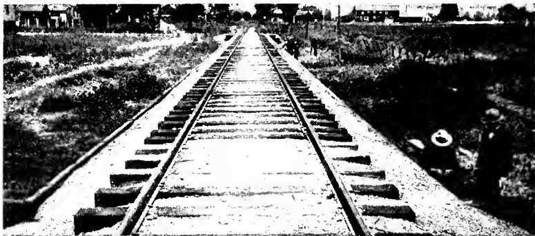
Picture 46. Trestle 45-E, Calistoga Line, Southern Pacific, 195 feet, CSB-4, built 1900 of creosoted Douglas fir. Photographed August 6, 1928.
