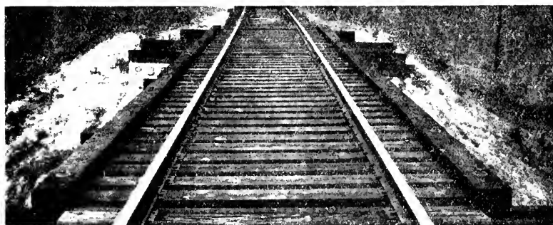
No. 20. C. R. I. & P. bridge 938, Haskell to Eldorado, Ark., constructed 1914, showing creosoted ties and 4-inch guard rails. Ties are spaced with creosoted wooden spacing blocks. Photographed May 24, 1928.
