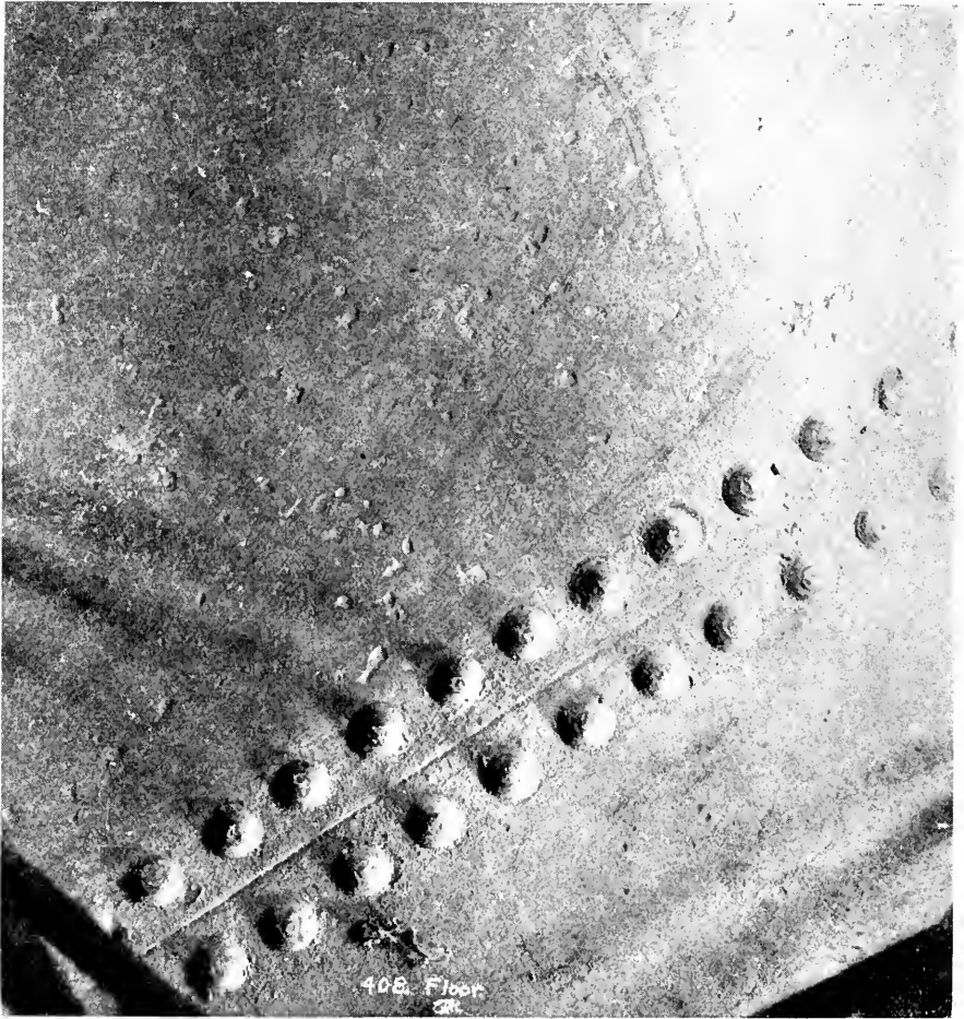
FIG. 3—INSIDE OF BOTTOM OF BOILER WASHING TANK AFTER TEN MONTHS' SERVICE. BEFORE BEING PLACED IN SERVICE THIS TANK HAD BEEN GIVEN TWO COATS OF PAINT ESPECIALLY RECOMMENDED BY THE MANUFACTURER FOR THIS SERVICE
