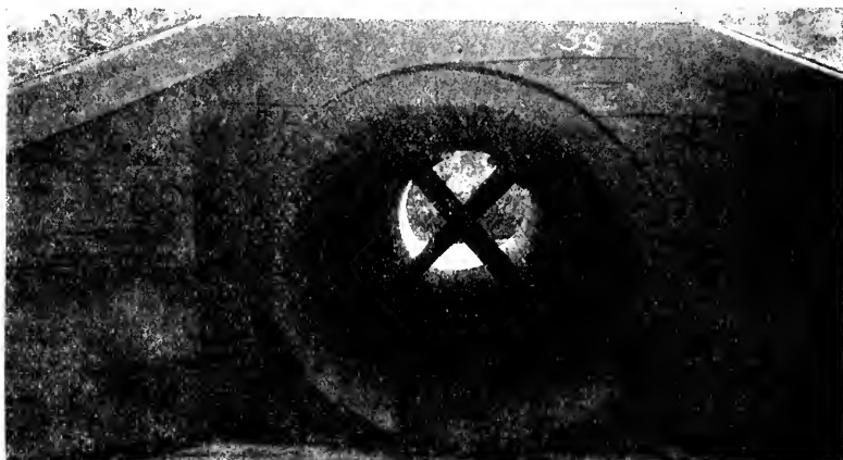
Picture 59. Creosoted wood stave culvert 56-G, Calistoga Line, Southern Pacific, built 1900 of creosoted Douglas fir. Staves are 4 inches thick—43 \frac{1}{2} inches and 5 \frac{1}{2} inches in width. Borings of staves and timbers of this culvert show sound timber. Culvert braced in middle as shown by photograph, some years after construction account crushing. Photographed August 6, 1928.
