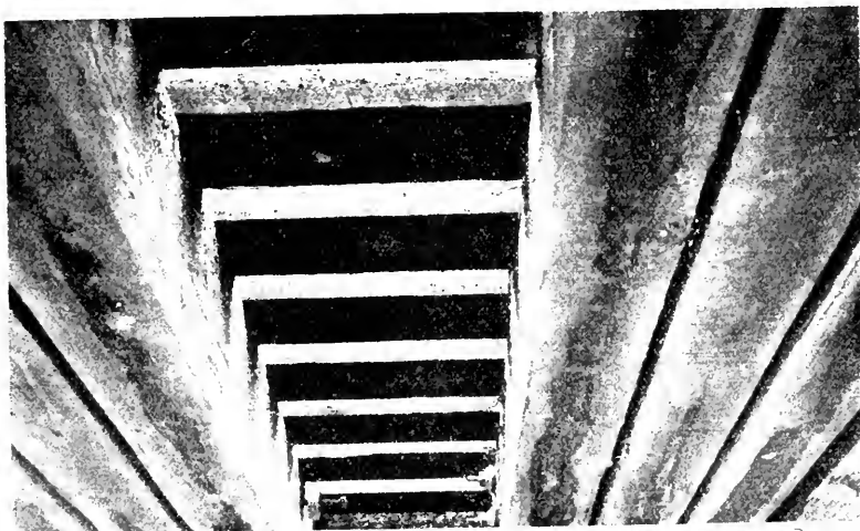
No. 11. C. R. I. & P. bridge 905, between Haskell and Eldorado, Ark., constructed 1914. View of creosoted Douglas fir stringers in place, since construction of bridge, all in excellent condition. Treatment approximately 7\frac{1}{2} pounds creosote per cubic foot. Hand adzing was done before treatment. Photographed May 24, 1928.
