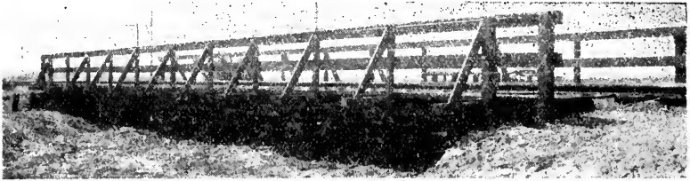
Picture 92. Trestle 468-A, Southern Pacific, east of Tejunga. Length, 75 feet, constructed of creosoted Douglas fir 1898. Six bents of four piles each. Two piles renewed in 1919. Also four caps have been renewed. Caps crushing under the head of the piles. Stringers are 12 x 12 laid solid. All timbers sound. Photographed August 10, 1928.
