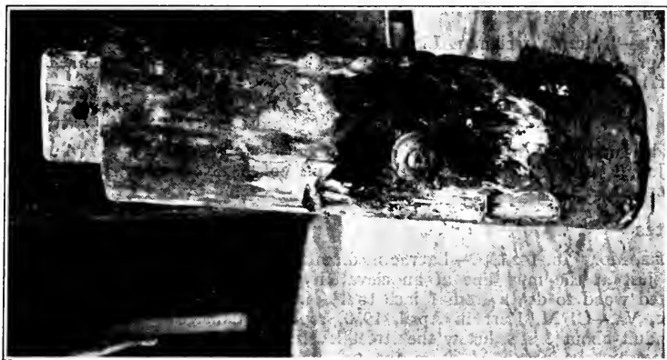
PHOTO No. 2.—Wharf Borer damage New York Dock Company, untreated pine pile, section above the water line.
