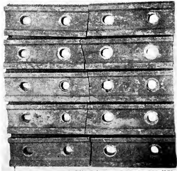
Fig. 4.—Typical Broken Bars Resulting From Progressive Fatigue Cracks Originating in Upper Contact Surface.
