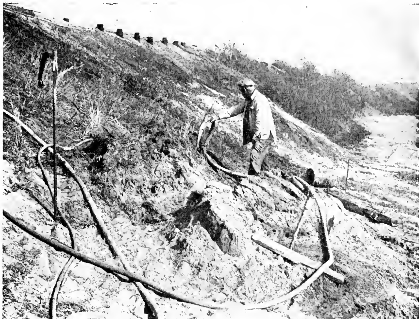
Fig. 11.—Fill Grouting on the Burlington, Red Oak, Iowa, Showing Pushup and Breakout.
