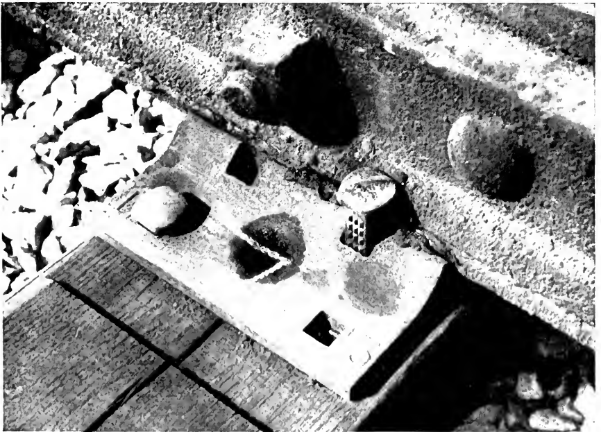
Fig. 8.—Section 7 on Curve with Two each of Racor Drive Tight Line and Anchor Spikes.
