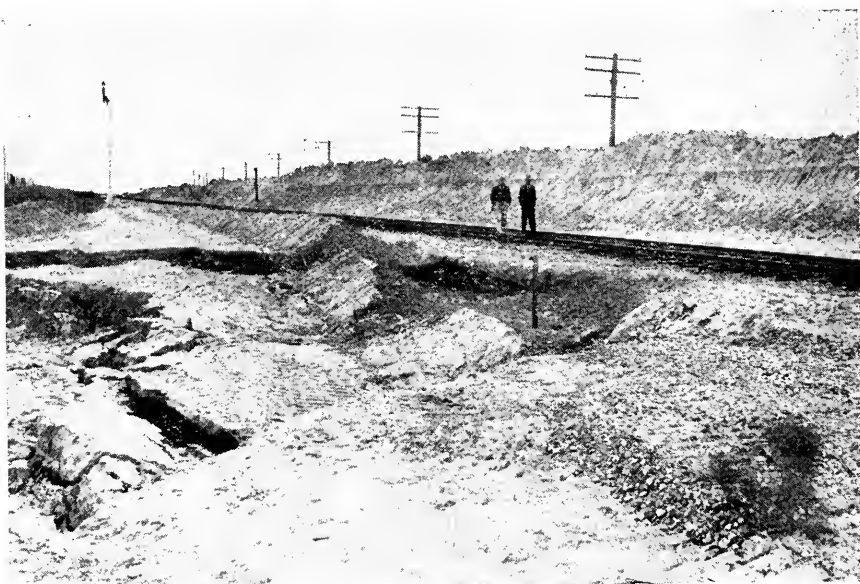
Fig. 13.—Slide in Silt Soils. Northern Pacific—Eastern Montana.
