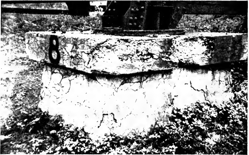
Fig. 1.—Disintegration of a Concrete Pedestal.
