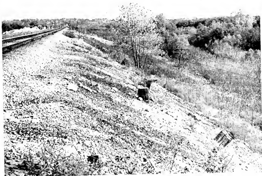
Fig. 10.—Displaced Piling on Sliding Fill. Burlington, Red Oak, Iowa.
