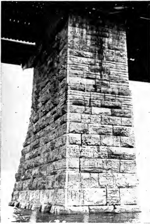
Fig. 7.—Vertical Cracks in this Old Pier Due to Progressive Increase in the Live Load.
