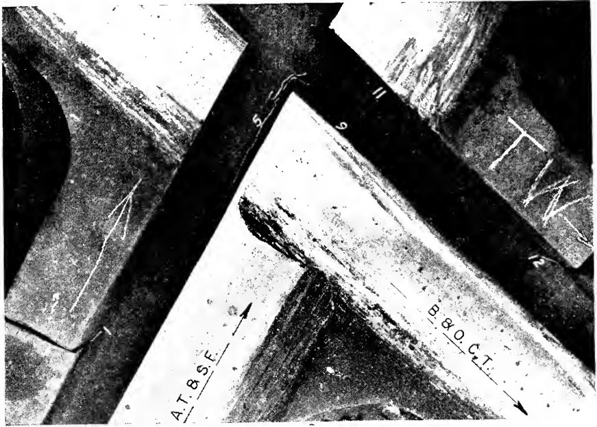
Fig. 1.—Original Taylor-Wharton Casting After One Year of Service. (Numbers in Flangeways Denote Stress Gage Positions).
