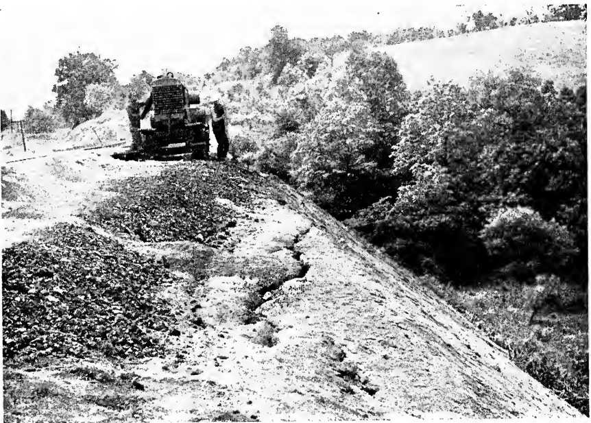
Fig. 4.—Unstable Fill Showing Shoulder Cracking. Wheeling & Lake Erie, Baltic, Ohio.
