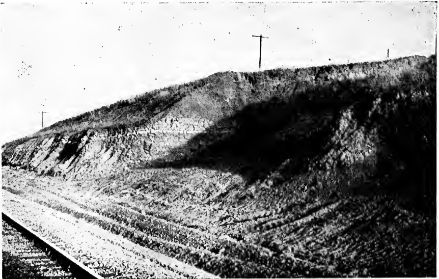
Fig. 7.—Unstable Cut Slopes and Berm. M-K-T R. R., Pottsboro—Sadler Revision.
