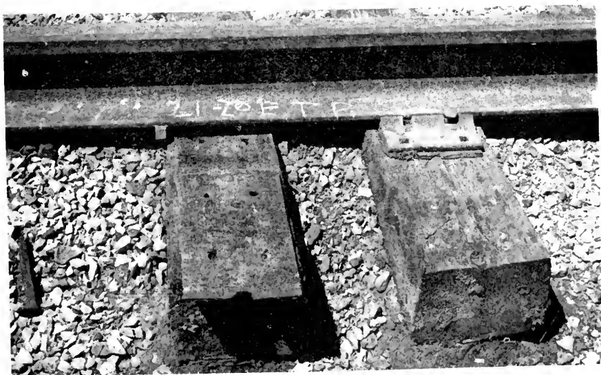
Fig. 8. Section 21, Fabco Pad (Uncoated) After 56-Months' Service in Tangent Track with Crec. Pine Ties.
