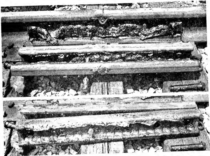
FIG. 13. Section 1, Filled with Gravel, Lubricated with Petroleum Grease and Plastic End Plugs.
