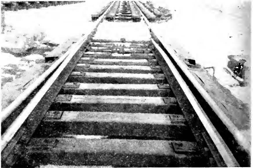
Fig. 5—End view of gas switch heater installation, which burns various types of gas, showing protecting shields.
