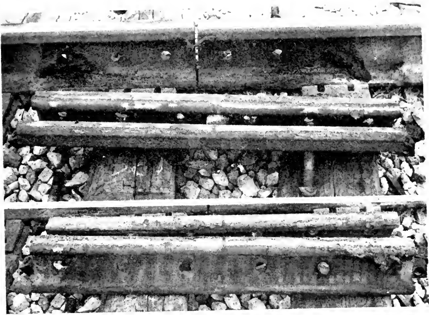
Fig. 9. North Portion of Section 4, No-Cx-Id "A" Special (Brush coat on rail and joint bars with No-Cx-Id End Plugs).
