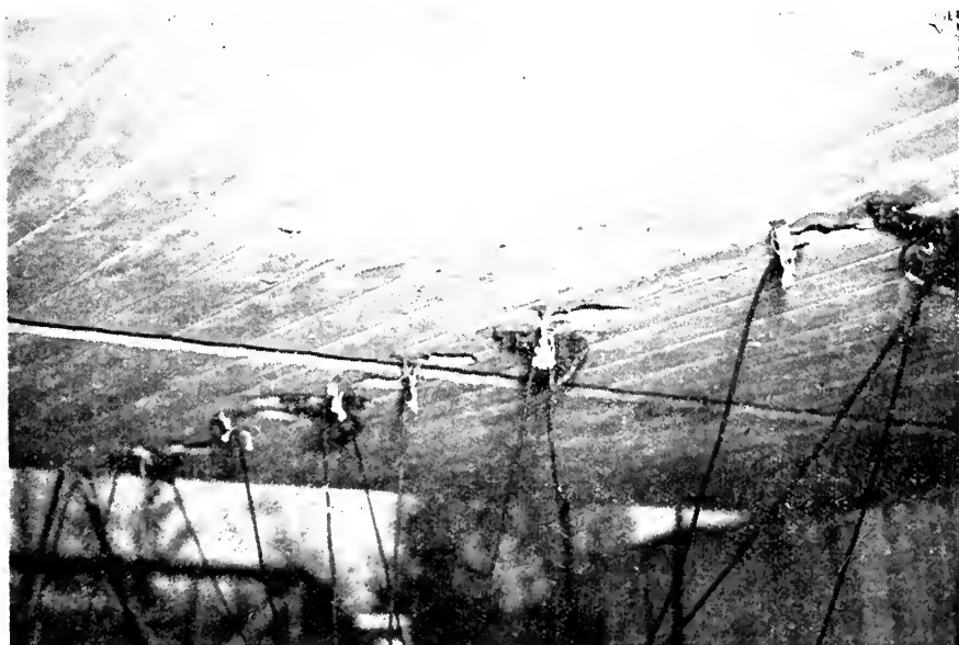
Fig. 4—General view of SR4 wire gages on reinforcing bars and electro-magnetic gages on concrete on bottom of slab.
