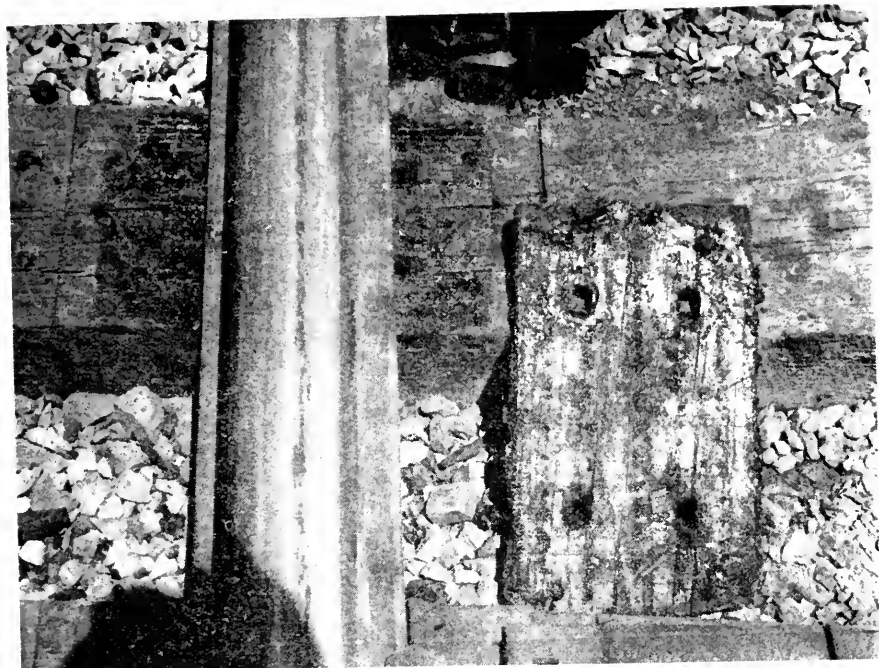
Fig. 7. Section 5, Bird 2-ply lock-belt pad (Section after 24 months' service in inner rail of long 4-deg. radius curve.
