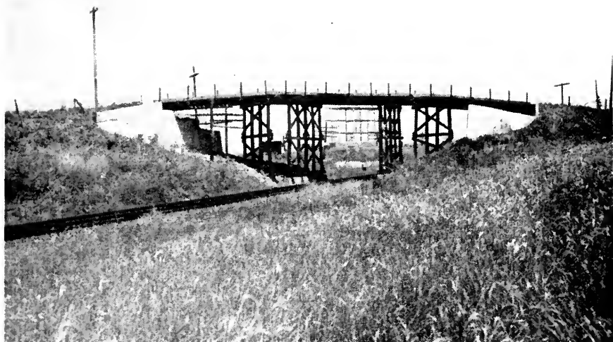
Illustration 8—View of the railroad structure where the 9-sq ft experimental panels were applied in July 1950. Wing walls of abutments shown have southerly exposure.
