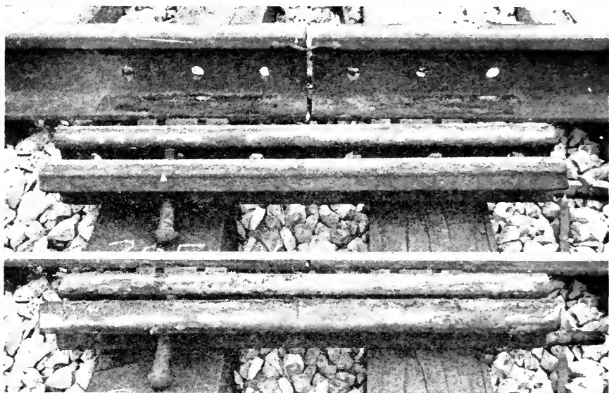
Fig. 7. North Portion Section 2, Bonoco Anti-Rust Compound (Brush coat on rail and joint bars).
