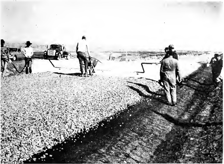
Placing cationic emulsion in the ballast in Section No. 6. The result is to produce a rubber-like cementing agent between the ballast particles.
