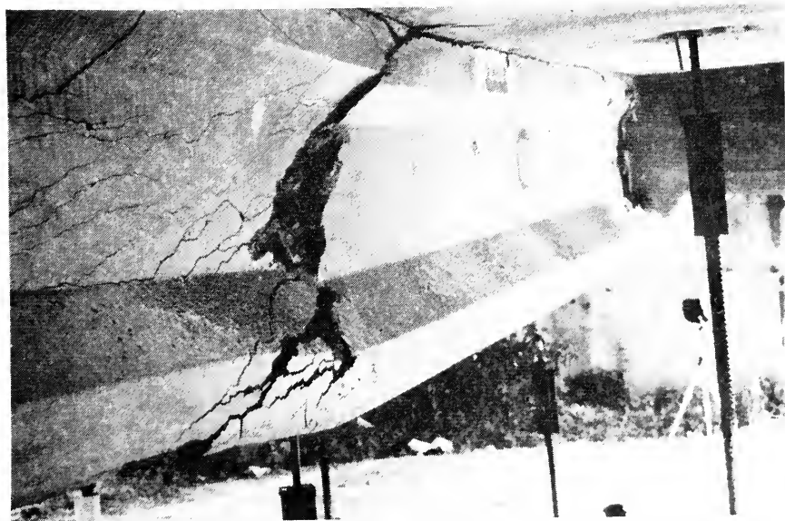
Fig. 10—Photographs illustrating mode of failure of Bridge 1 (above) and Bridge 2 (below).
